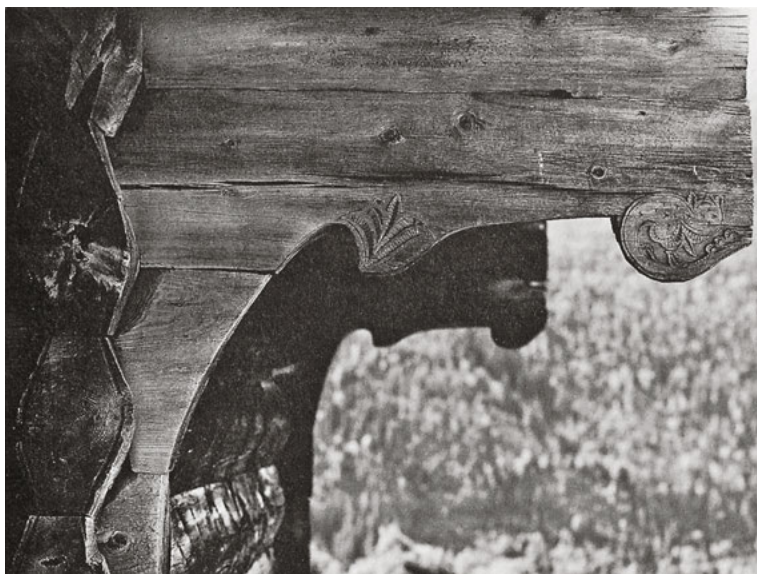
124 These rainwater drips on the jettied timbers of this loft in Øverbø, Telemark, Norway, are so beautifully decorated that it is easy to overlook their real function.
