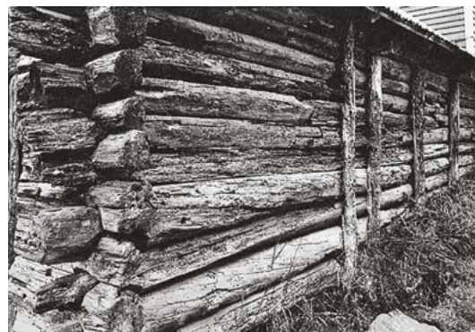
21 There is not a single log on this barn in Solvorn, Sogn, Norway, which is not severely damaged.
