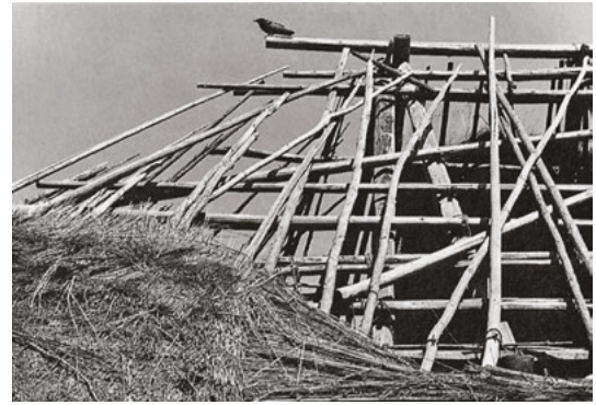
77 Spar roof construction of a minka exposed to decay. – Ayaori, Iwate, Japan.
