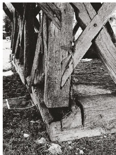
16 The thrust of the corner column of this bell tower in Malé Ozorovce, Slovakia, exacerbates the rotational movement of the twisted-fibre sill beam. As the halved-and-tabled joint prevents it from deflecting, it has to split.
