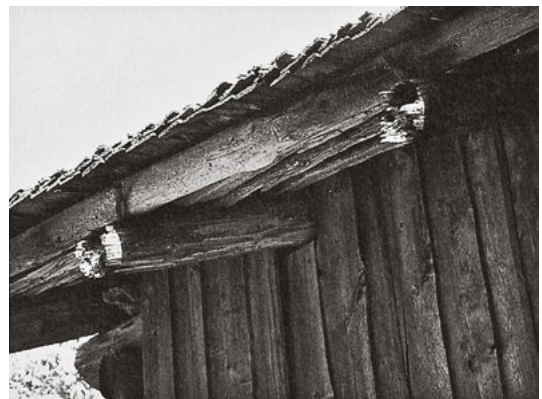
34 The rafters of this barn in Galgenuel, Vorarlberg, Austria, demonstrate quite clearly wood's weakest point.
