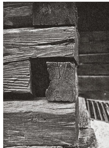
191 Due to the warping of the whole log, the joint on the end of the log has broken off the piece of wood which hides the notching and hence negated its purpose.— Church in Hervartov, Slovakia
