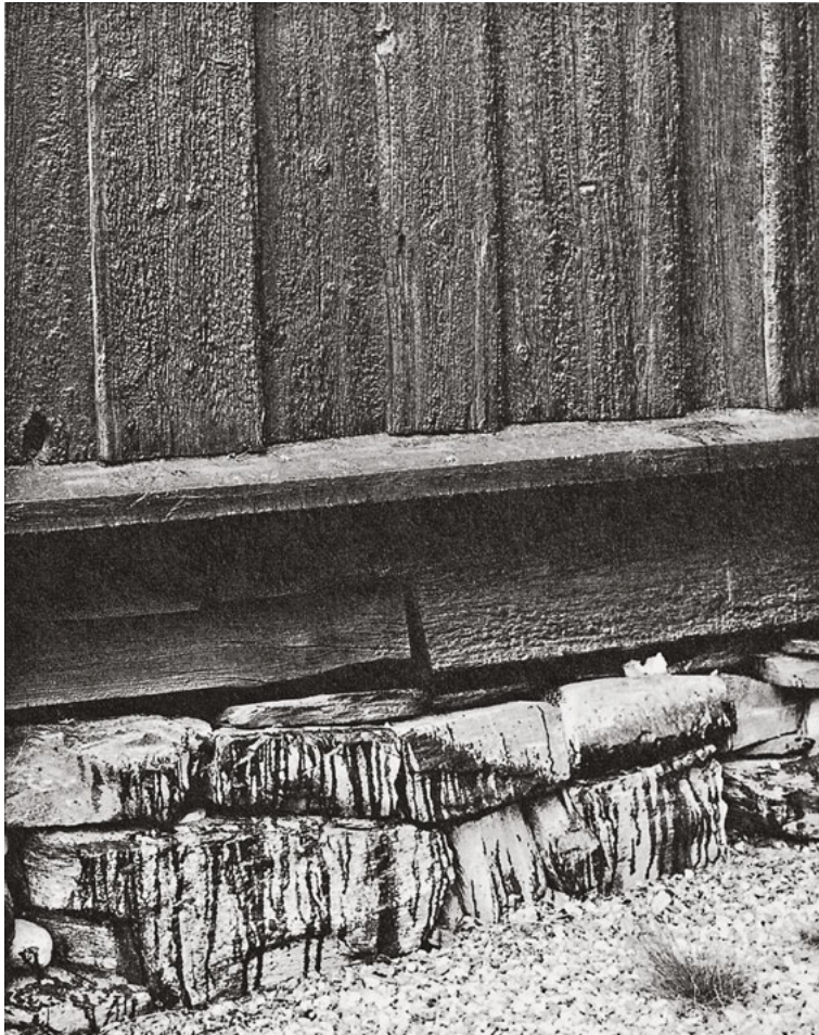
201 If this unkeyed tabled scarf joint on the sill beam under the svalgang to this stave church manages to fulfil its purpose, it is not thanks to the carpenter! – Ringeby, Oppland, Norway
