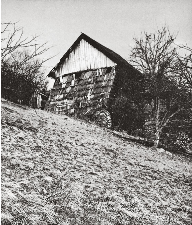
318 A log building which has lost its equilibrium is extremely unstable. – near Javorina nad Rimavicou, Slovakia
