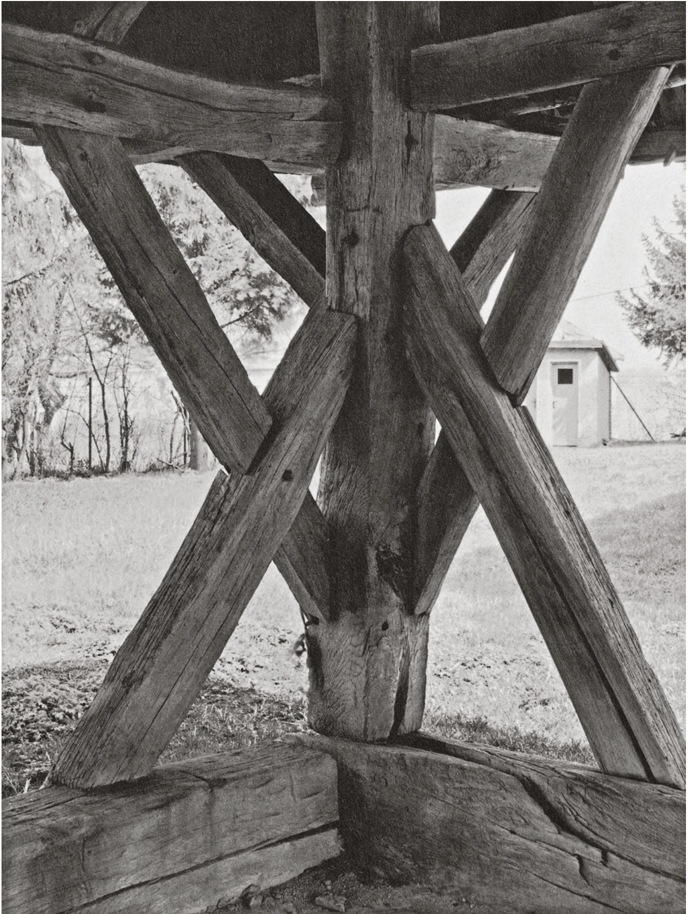
188 The corner of the bell-tower in Malé Ozorovce, Slovakia. The thrust of the inclined column has split apart the poorly selected sill beam to a worrying degree.
