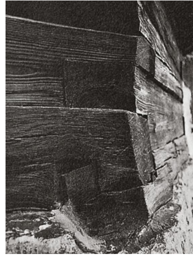
299 The sill beam of the church in Hervartov, Slovakia, has twisted out of its joint despite the weight of the whole church resting on it!
