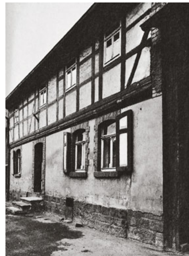
57 This plastered false wall concealing the timber-framed wall in Berga, Thuringia, Germany, allows water to collect exactly where the ends of the beams of the jettied upper floor are supported.
