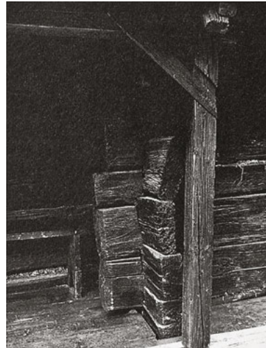
307 "Bulging" describes superbly the buckling of these logs on the church in Topola, Slovakia.
