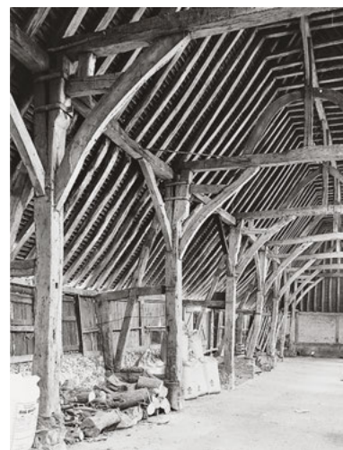
112 Iron straps prevent the worst in this barn in Frindsbury, Kent, England. The thrust of the roof has split open the columns via the tenons fitted into the header beam and against the tension of the tenons fitted into the tie beam.
