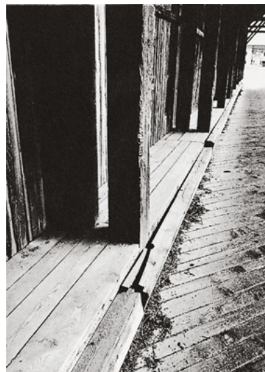
15 Even sophisticated timber joints would not have been able to prevent this timber from twisting. – Wooden bridge in Umhausen, Tyrol, Austria.
