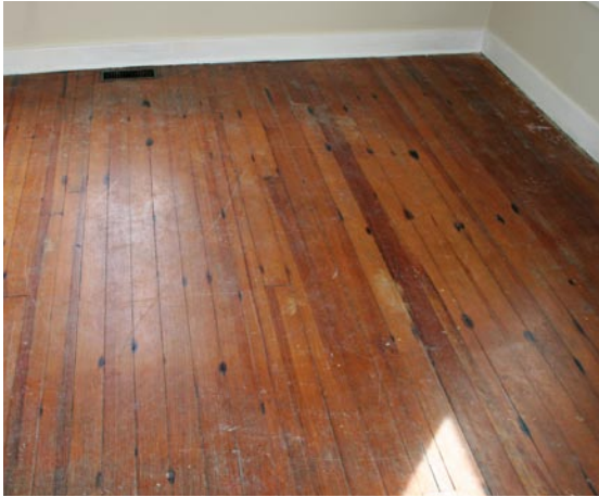
Iron stains are visible near the nail locations.
