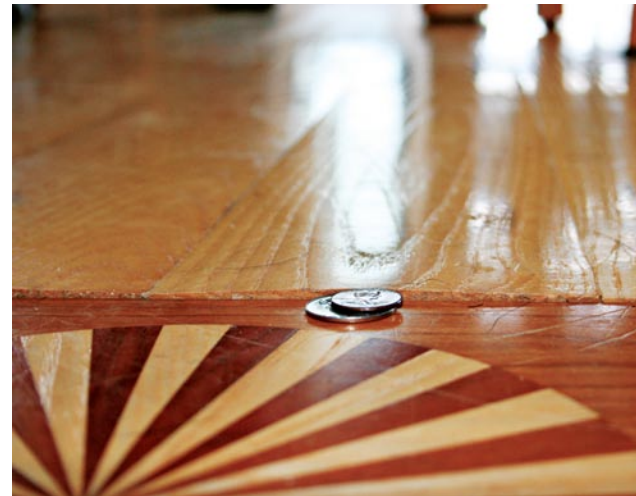
Centers of crowned floorboards are higher than the edges.
