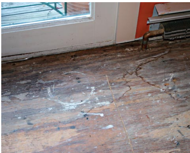
Water stains on the subfloor are a telltale sign of leaky doors and windows. Be sure doors and windows are properly flashed so as not to leak before installing a wood floor.
