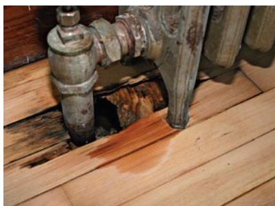
Punky, rotted wood can happen to the best of floors.
