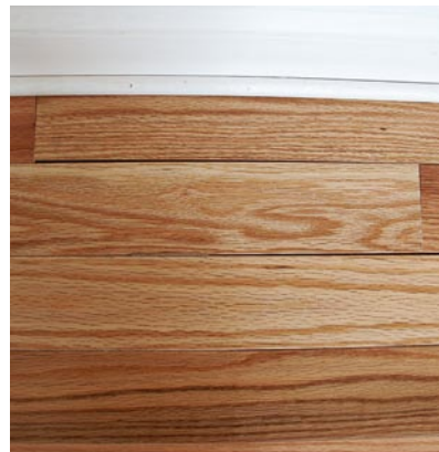
Other gaps are the result of poor installation techniques.
