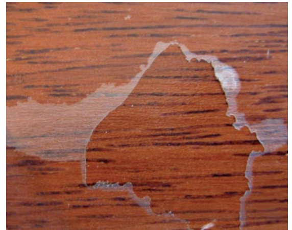
Peeling finish: The finish separates in sheets or strips from the flooring or from an underlying coat of finish.
