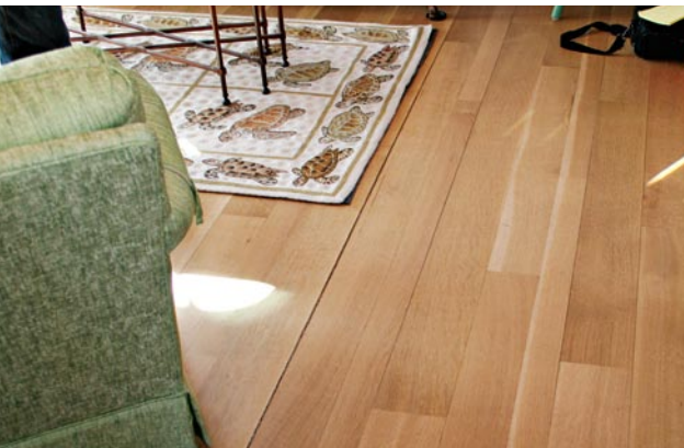
A gap above a floor beam runs the length of the room.
