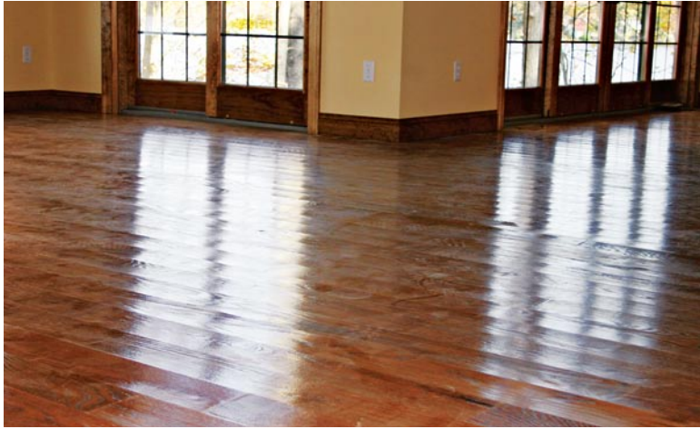
Cupped floorboards are higher at the edges than at the center.
