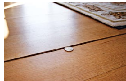
Overwood is when the edge of a board is higher than an adjacent one.
