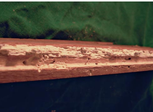
Powder-post beetles can cause severe damage to sapwood.
