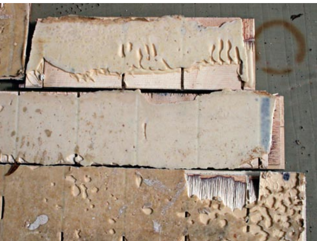
Adhesive failure occurs when glue-down flooring separates from its subfloor or concrete slab.
