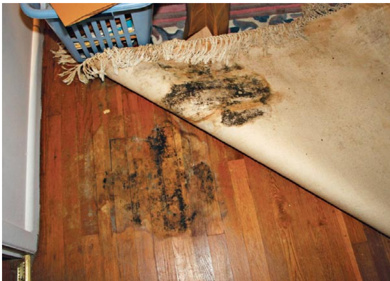
Mildew stains require prolonged levels of high moisture.
