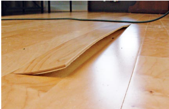
Delamination: The veneer layer separates from the substrate of engineered flooring.
