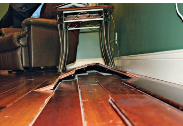
Buckling and bridging: Sections of flooring raise off the subfloor, pulling nails or breaking adhesive bonds.
