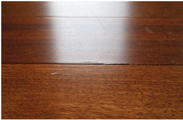
Fractures on prefinished board edges: Damaged wood or finish along the tongue edge of nailed-down prefinished flooring.
