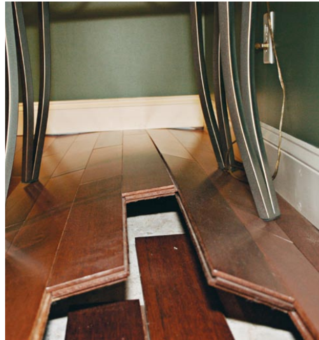
When wood flooring expands due to moisture absorption, it can push hard enough to move walls and crush the edges of boards that are capable of withstanding 1,000 lb. per sq. in. of pressure.
