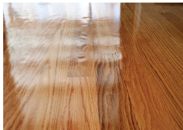
Dishing: Softer areas of the floorboards are lower than harder ones.
