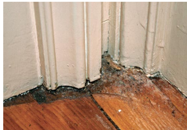
Corners not scraped occur when areas where the machines cannot reach are not sanded.
