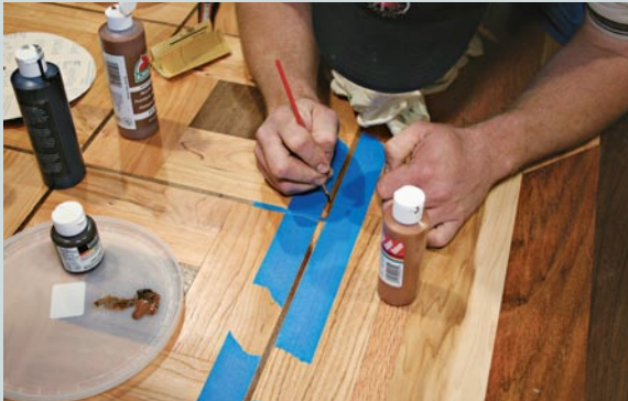
Carefully mask the damaged area, and blend acrylic paint to color-match the damaged strip in the floor.
