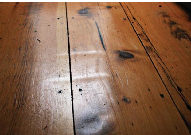
Drum marks are hollows in the floor that mirror the shape of the sanding drum.
