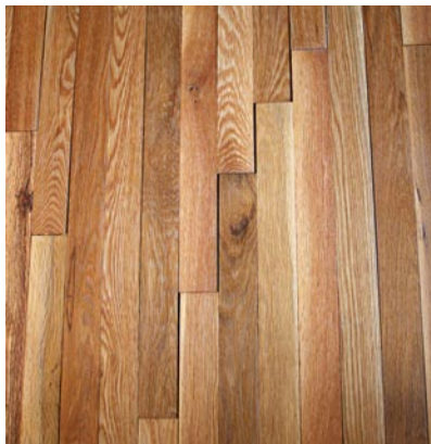
Gaps from cross-pull appear in a staircase pattern.
