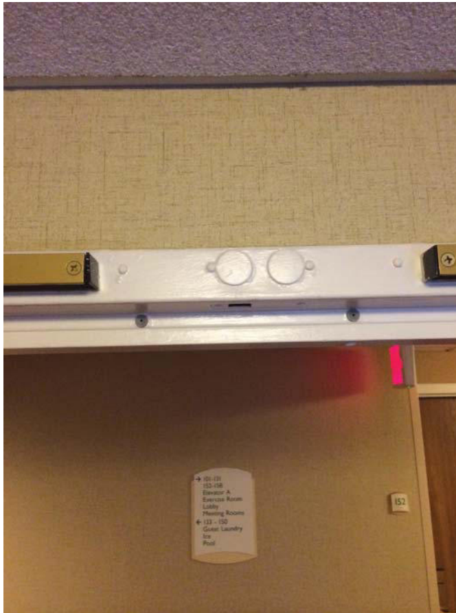
FIGURE 9.47 Pair Metal Door Frame Silencer Installed
