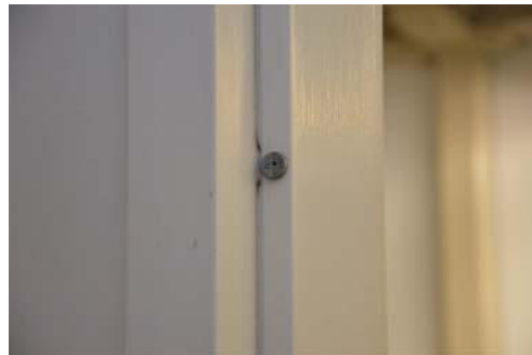
FIGURE 9.46 Pair Metal Door Frame Silencer Installed Close Up (Source: Courtesy of Scott J. Tobias)
