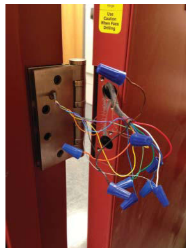
FIGURE 1.36 Electric Transfer Wired to Door
