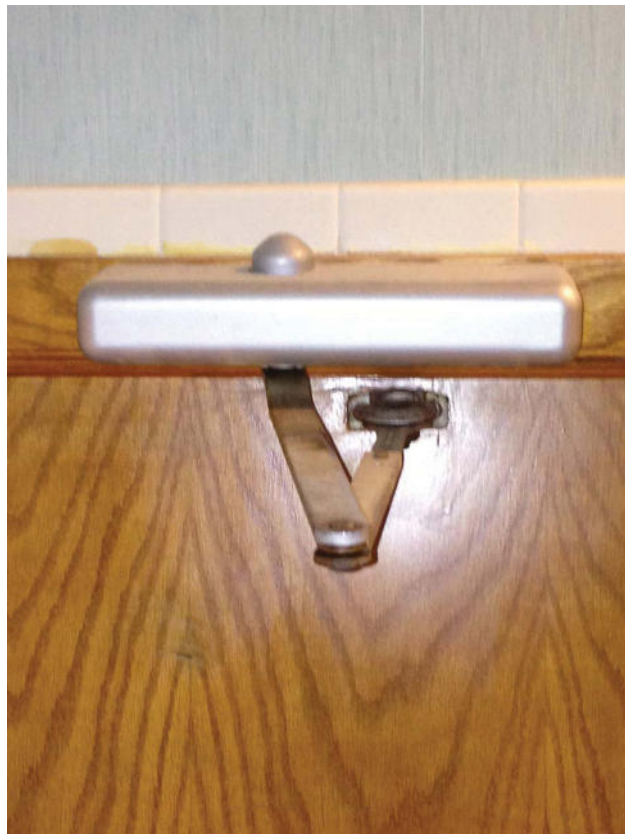
FIGURE 5.10 Regular Arm Door Closer Not Installed Properly (Source: Scott J. Tobias)
