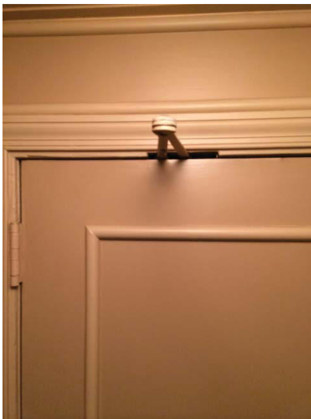
FIGURE 5.11 Door Closer and Door Molding Conflict
