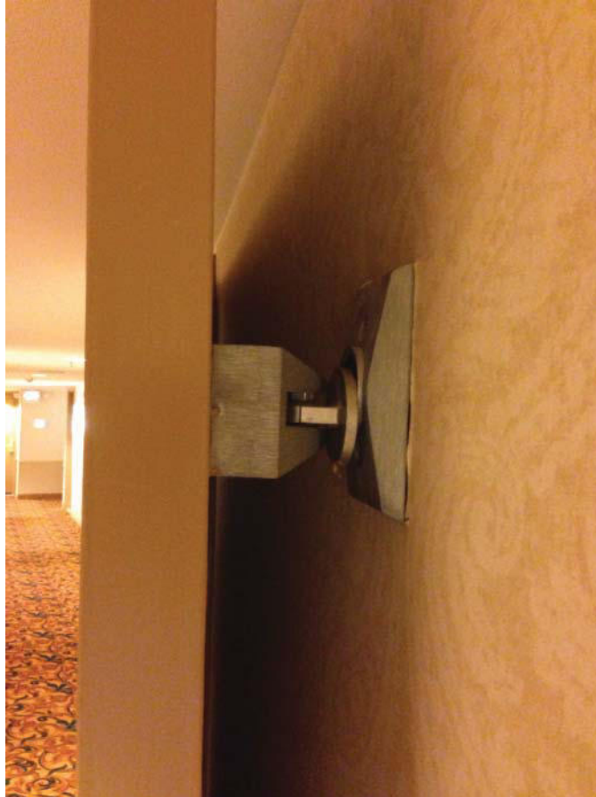
FIGURE 7.8 Electromagnetic Hold-Open Not Aligned Properly (Source: Courtesy of Scott J. Tobias)
