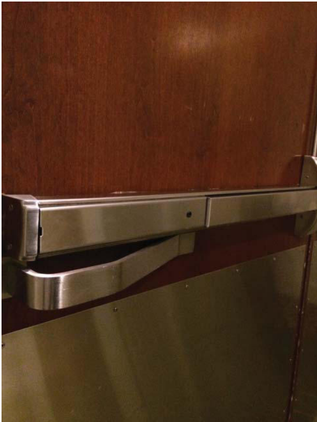
FIGURE 9.1 Exit Device Bumper Guard (Source: Courtesy of Scott J. Tobias)
