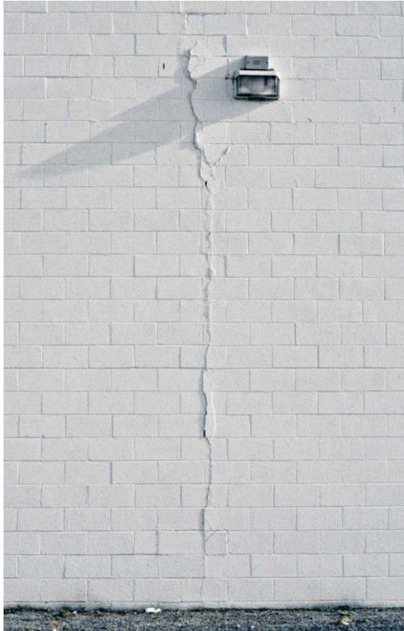
THIS WALL MADE ITS OWN CONTRACTION JOINT. Quarter-inch contraction joints made of a high-grade elastomeric sealant allow a block wall to shrink, instead of crack, as water dissipates from the grout. This wall should have had these control joints every 15 ft. to 20 ft.
