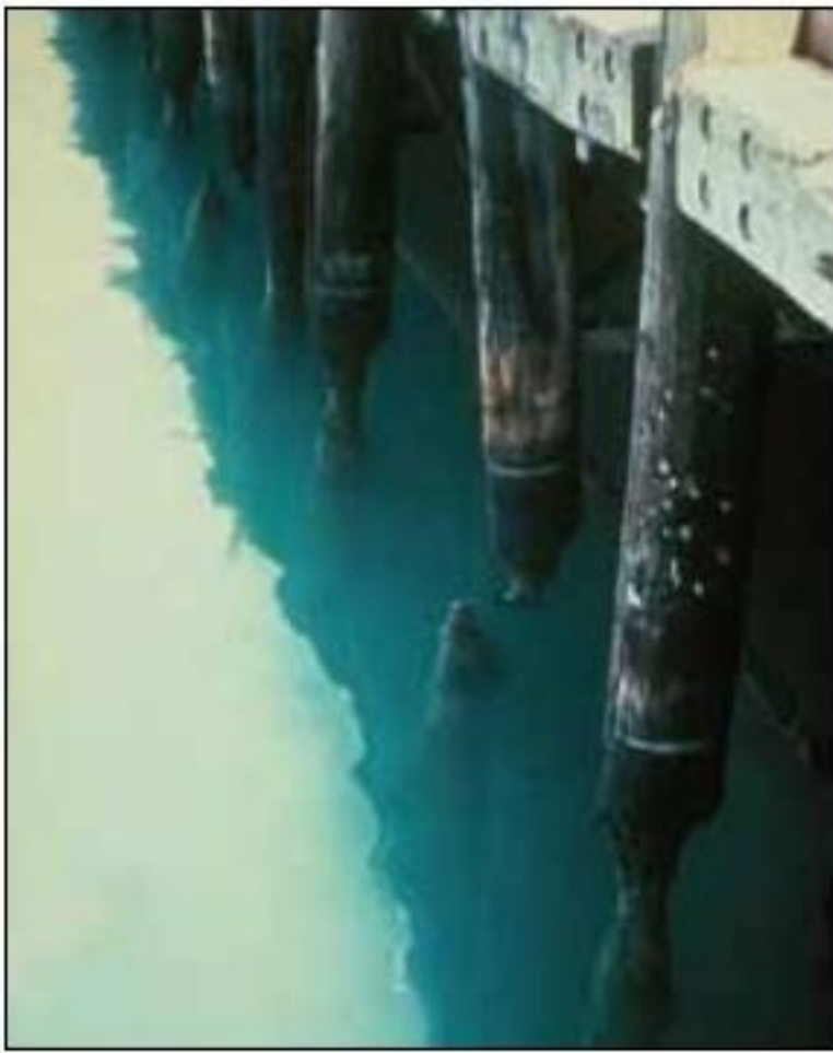
Figure 14–11. Limnoria damage to piling.
