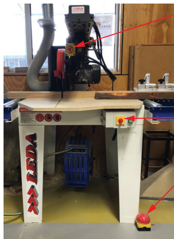
Fig. 11.1 Emergency stop switches
