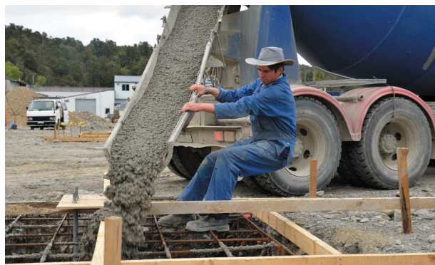
Fig. 31.24 Site delivery chute
