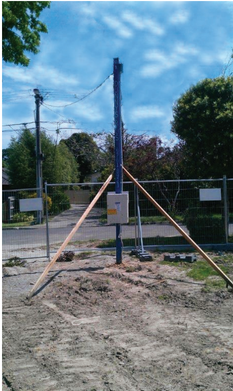
Fig. 10.1 Domestic temporary power pole
