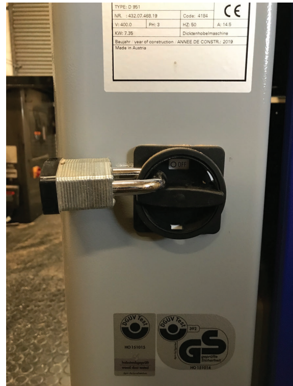
Fig. 11.2 A padlock used to lock off an isolation switch
