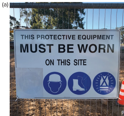
Fig. 3.9 (a) and (b) Safety and warning signs
