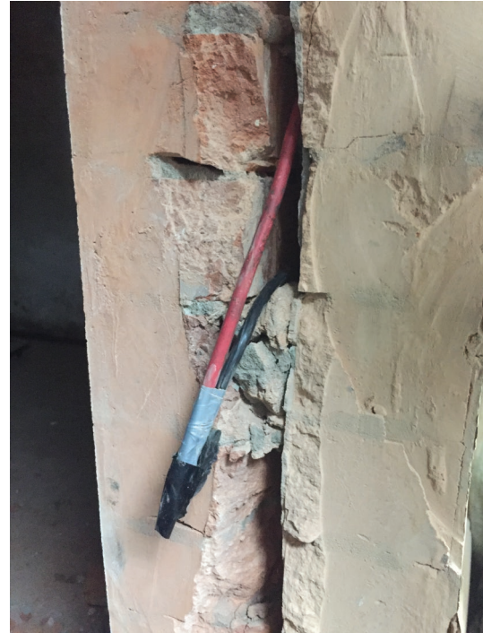
Fig. 34.4 A near miss that could have been deadly: these wires were disconnected, taped and pushed back into the brickwork cavity during a previous renovation. The demolition saw was only millimetres away from cutting through them. A licensed electrician was immediately brought in to fix the situation
