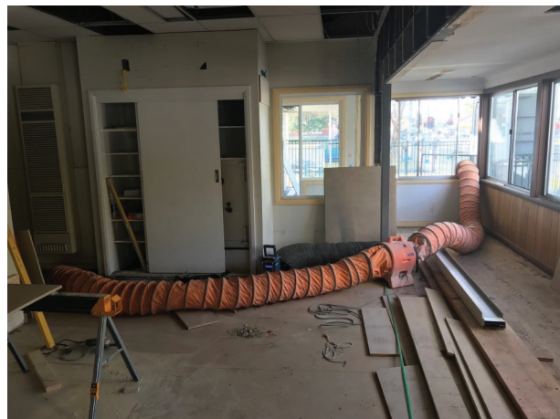
Fig. 34.17 Industrial exhaust system for the removal of dust
