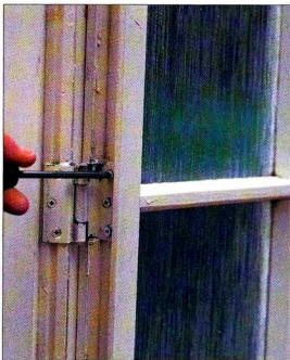
Above A binding window may be cured simply by tightening the hinge screws or replacing them with longer ones.
