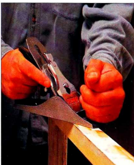
Above A sticking window may be swollen or have too much paint on it. Plane down the leading edge of the window.
