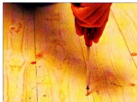
Above Secure loose floorboards by replacing the nails with screws.
