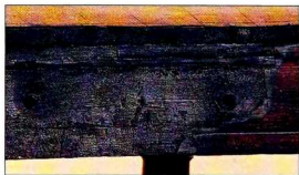
Above Burn damage
