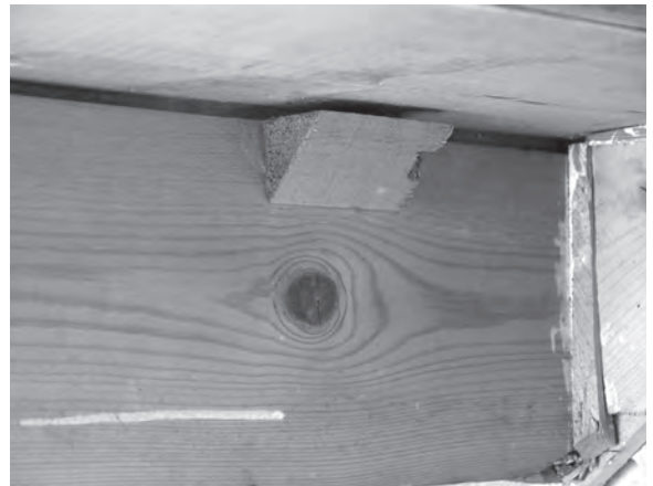
Figure 12.2 The movement of this tread as the gap closes under the weight of a stair user results in loud and unwanted creaking.
