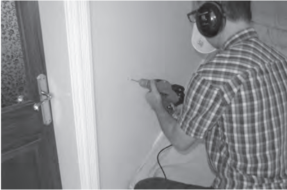
Figure 12.72 Always beware hidden services when drilling into a wall.
