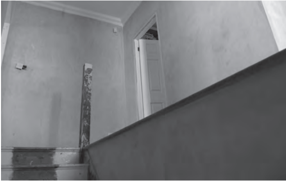
Figure 12.45 Along the landing, a new horizontal balcony balustrade is required.
