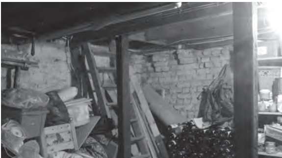
Figure 4.3 A wooden ladder propped against a wall is not the safest way to access a cellar.
