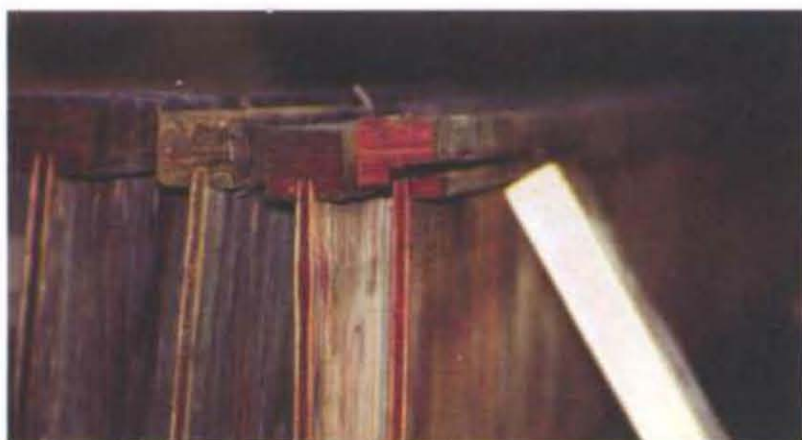
Damaged flanges can cause I-joists to fail. Carefully check the joists before installation and handle with care on site. (Photo by Roe A. Osborn, courtesy Fine Homebuilding magazine, © The Taunton Press, Inc.)
