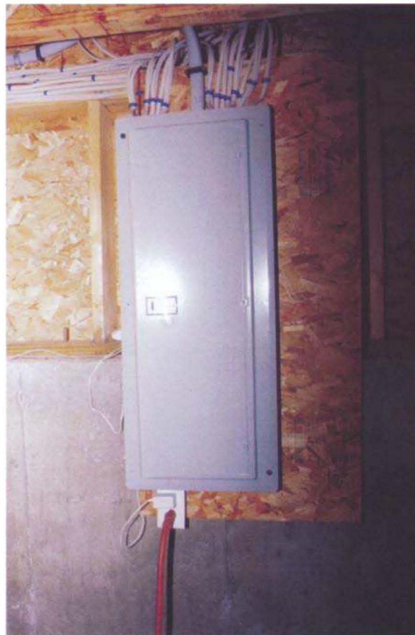
The electrician needs a solid backer on which to mount the electric service panel.
