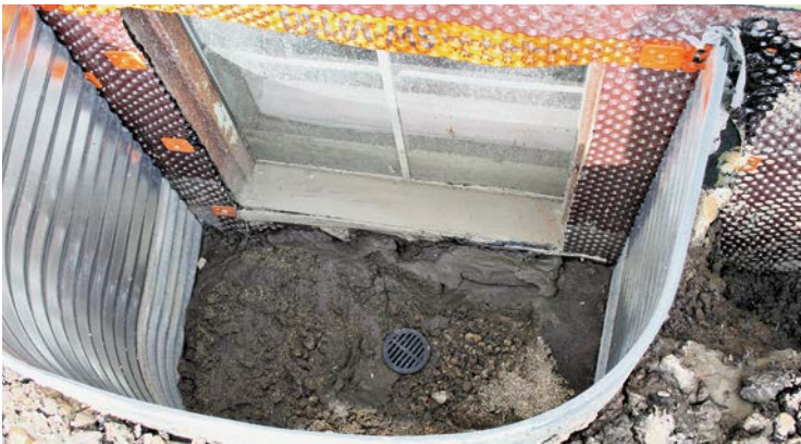
This window has a rusty metal frame, which can be repaired by painting with rusty metal primer, then a finish coat. The area around the frame has been filled with caulk and covered with waterproofing fabric. A gap at the bottom has been filled with mortar.
