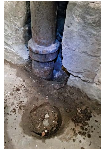
An old cast-iron drain stack with a cleanout at the floor will likely be rusted; it is usually a good idea to replace the cleanout and some of the pipe.
