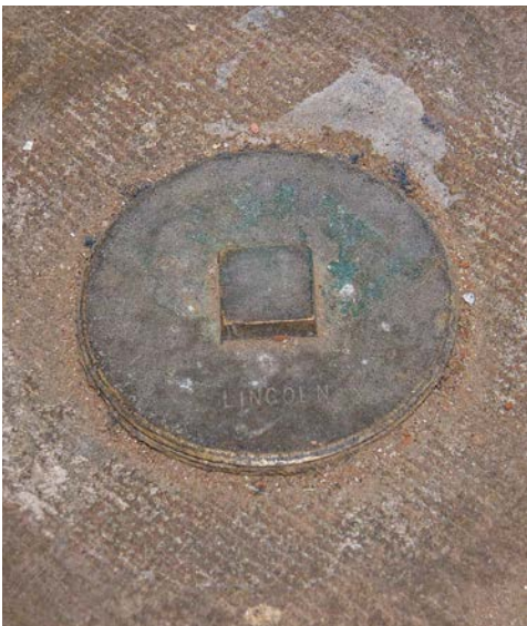
If you see a cylindrical fitting under the floor, like this brass cleanout, you have an old-fashioned drum trap. It will likely last, but it would be better to tear up the floor and replace the fitting with a P trap. In any event, if you install flooring here, be sure to provide access to this fitting in case you need to rod the drain line in the future.
