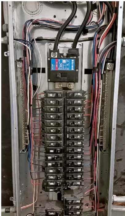
A well-organized service panel has wires that are neatly routed to their breakers.
