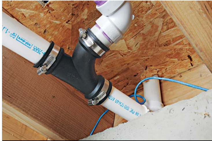
6b . . . and also to a house vent.
