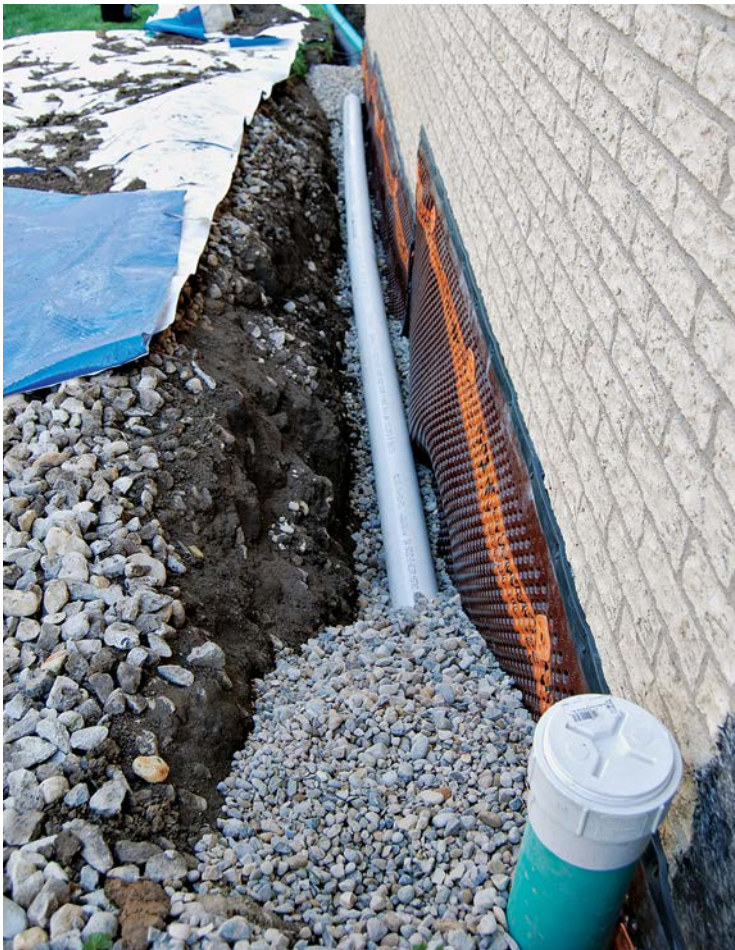
If you are going to the trouble of digging a trench down below the top of the footing, the fix should be done right.
