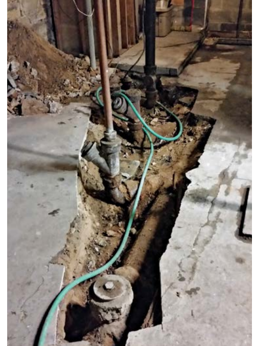
When running new drain lines into an existing old main drain, it's a good idea to chip away the concrete and find out the condition of the pipe. You can see plenty of rust, which is partially encased in concrete and will some day cause the pipe to fail. This should be replaced with PVC piping.
