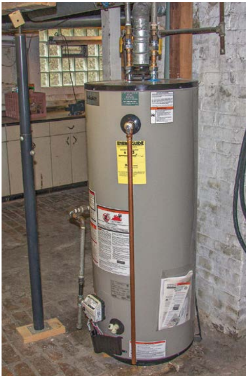
A standard tank-type water heater like this is still the most common choice. If your family sometimes runs out of hot water, consider buying a new unit with a larger capacity.
