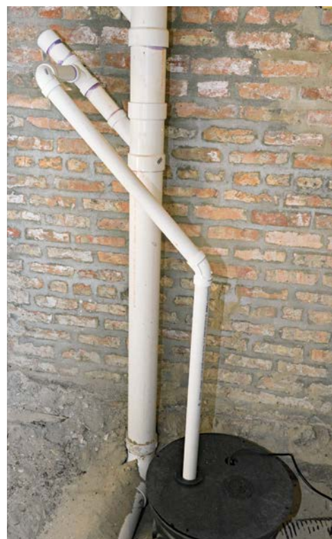
In this installation, the sump pump's drainpipe runs into the house's drainpipe.
