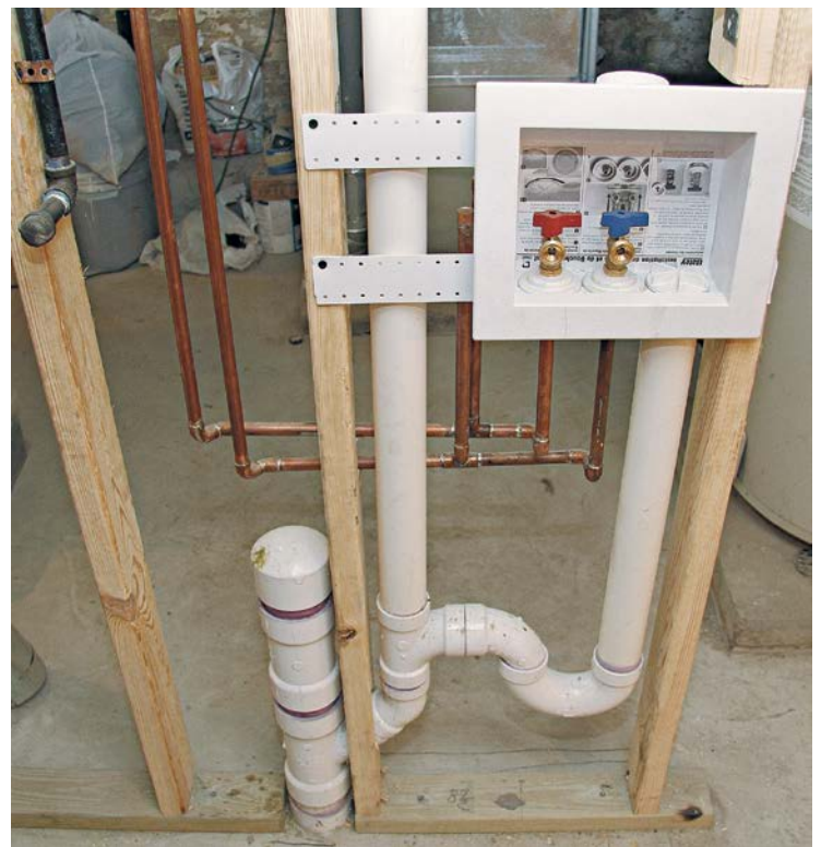
A washing machine outlet box includes a shutoff unit with a single control for both hot and cold water, as well as an outlet for the washing machine drain hose. At left you see a gas pipe for a gas dryer.
