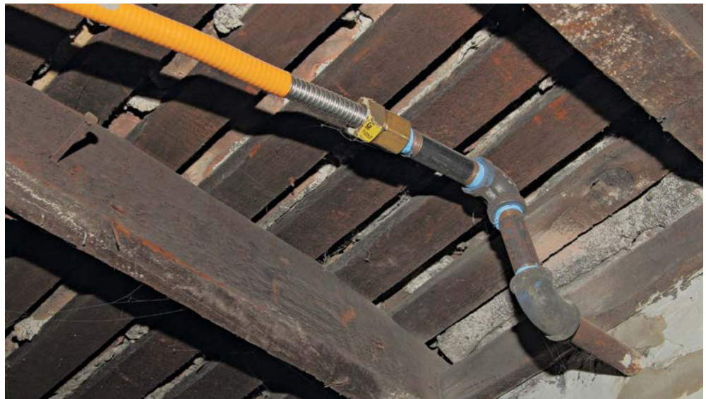
This gas line looks unusual but is actually just fine, though it may not be up to local code. Although the gas pipe is a bit rusty, it is not in danger of failing. Blue Teflon tape at the fittings is approved for use on gas lines.
