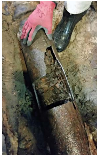
This main drain is almost completely clogged, which is not that unusual in an older home.
