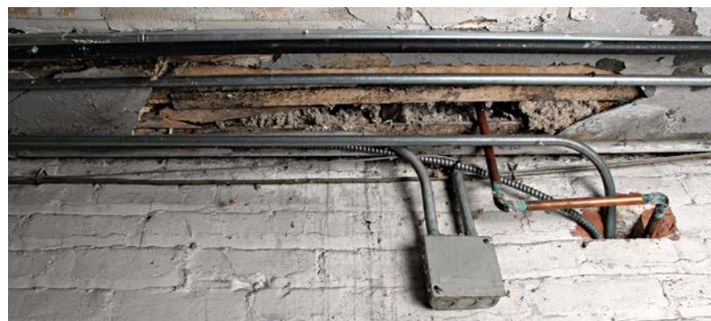
This tangle of tubes includes electrical conduit and cable as well as a black gas pipe and water supply pipes in copper and galvanized steel. Galvanized pipes almost always should be replaced. In this case, the copper pipe shows signs of decay as well.
