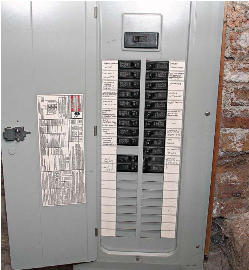
The electrical circuits in this service panel are neatly labeled, so if one overloads, you can easily find the breaker to flip. Also, there are many available slots for installing new circuits, which you will likely need when remodeling a basement.
