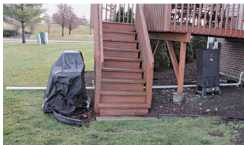
The sump pump's drainpipe runs outdoors.
