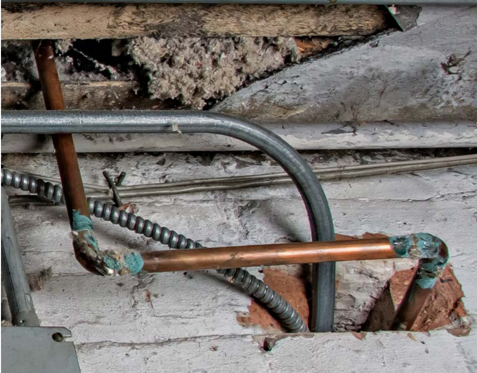
The green bubbles and stains on this copper gas pipe mean that moisture has been allowed to collect. This type of gas pipe installation is no longer up to code and needs to be replaced with approved gas pipe.
