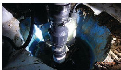
The sump pump issues were just the beginning of what this family had to deal with in the wake of Hurricane Joaquin.
