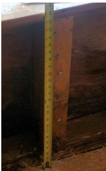
Measuring how far the water damage spread.
