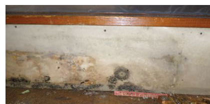
Crews found mold in parts of the home.
