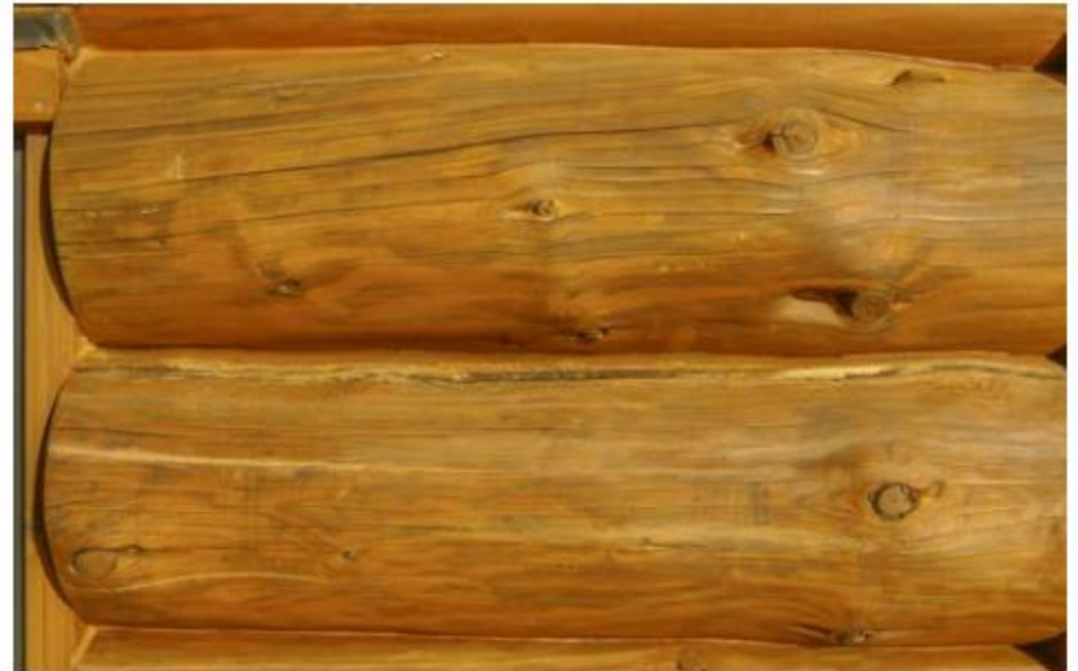
Upfacing check (crack) with signs of rot.
