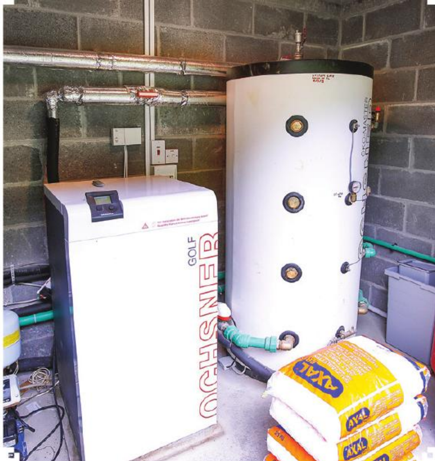
Heat pump with thermal store
