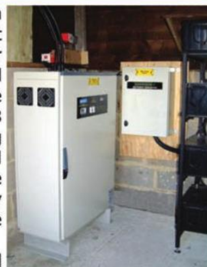
PS SYSTEM INSTALLATION
