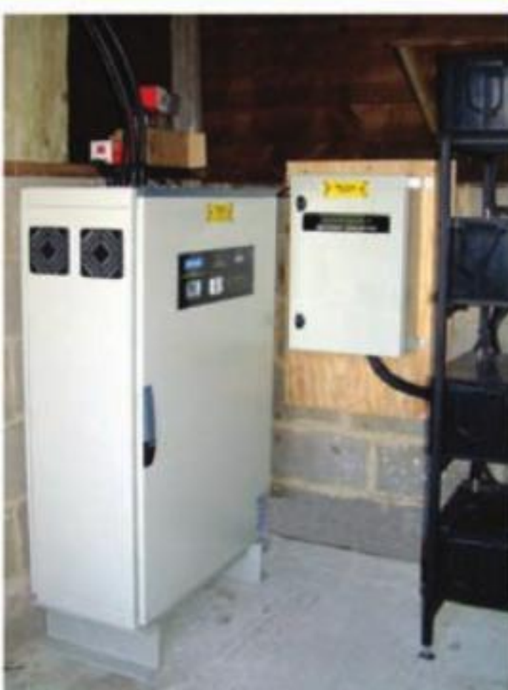
PS SYSTEM INSTALLATION
