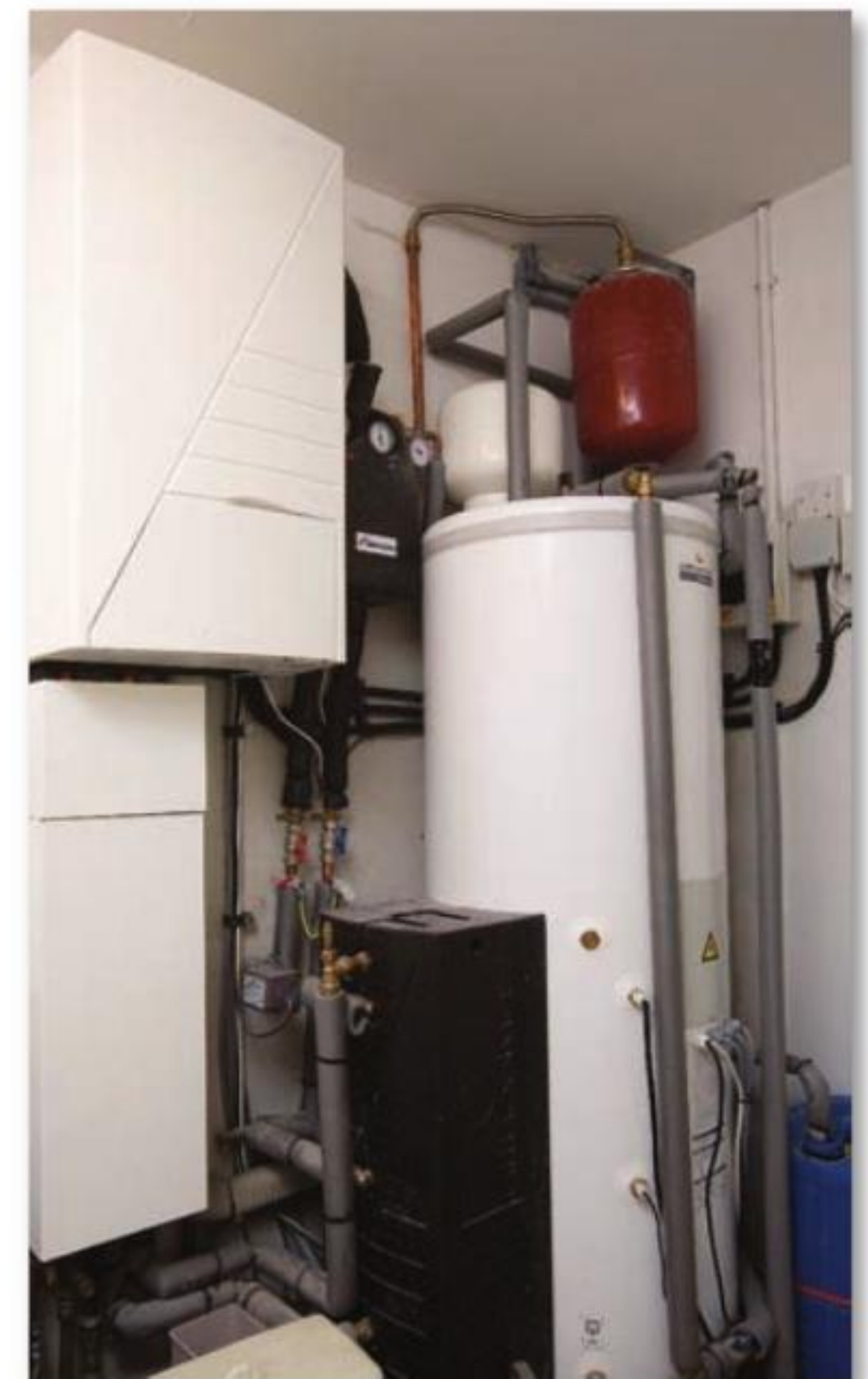
THE OPERATIONAL END OF THE RAINWATER RECYCLING AND AIR-SOURCE HEATING IS TUCKED AWAY IN THE UTILITY ROOM
