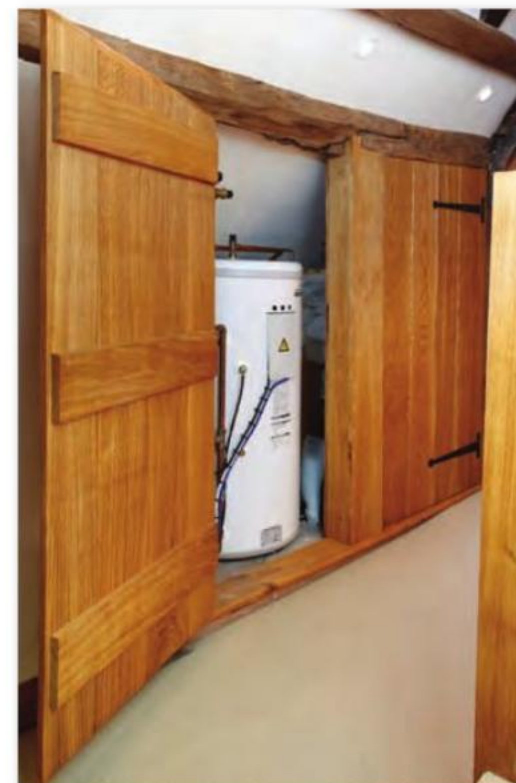
THE CENTRAL HUB OF THE HOME IS THE HEATING AND HOT WATER SYSTEM
