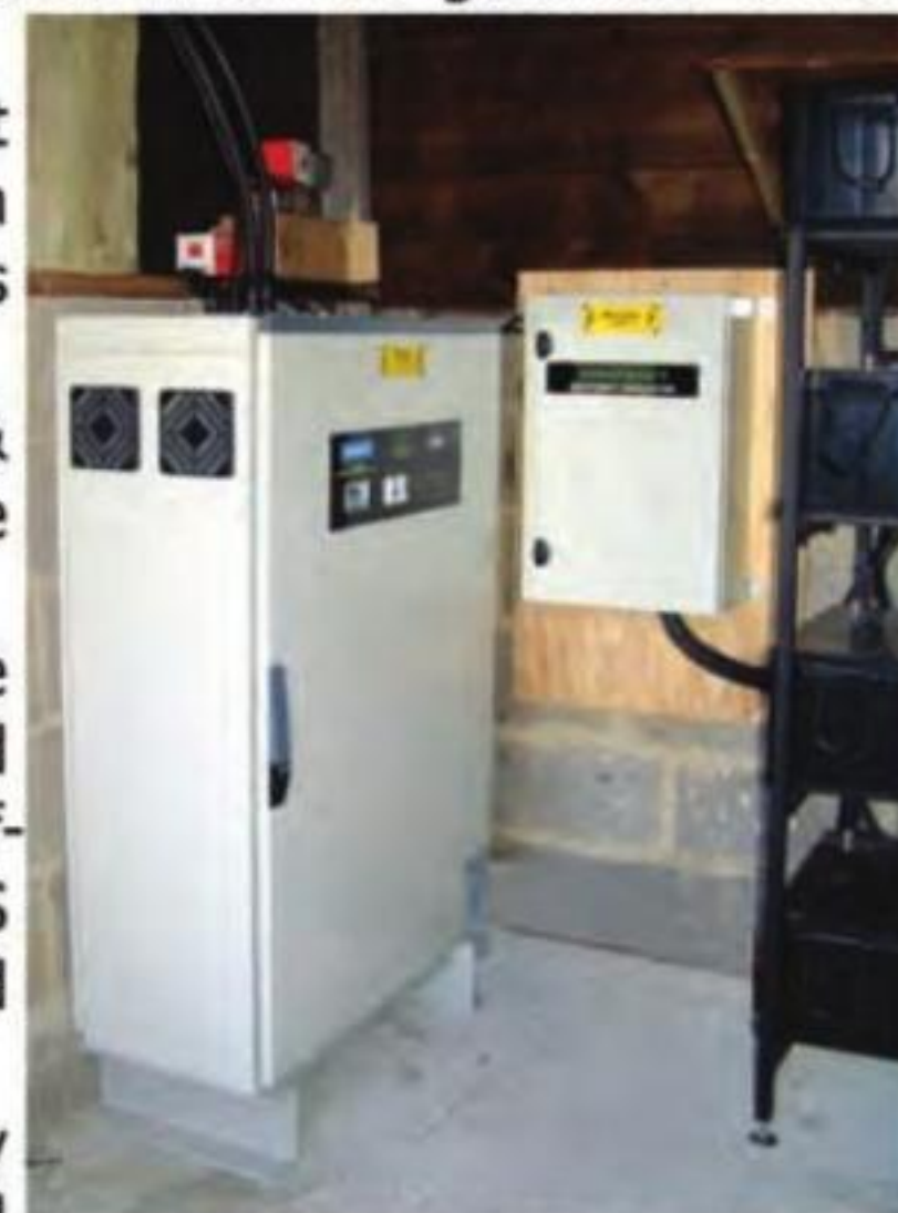
PS SYSTEM INSTALLATION
