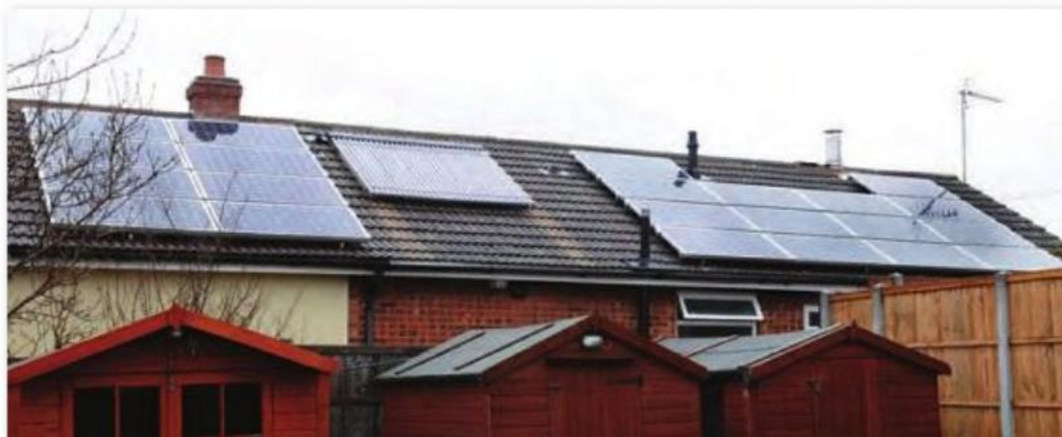
A TYPICAL DOMESTIC SYSTEM CAN SAVE APPROXIMATELY 1.2 TONNES OF CARBON DIOXIDE PER YEAR
