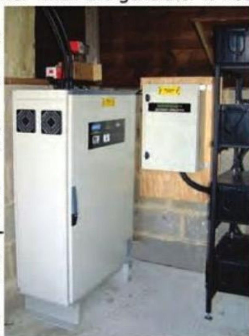
PS SYSTEM INSTALLATION
