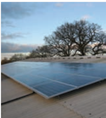
SOLAR PV PANELS ON A NEARBY BARN HELP ELIMINATE ENERGY COSTS
