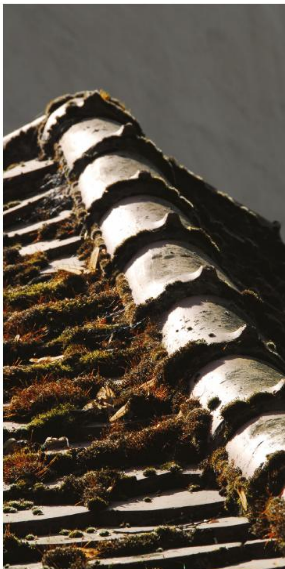
Left: Moss can lead to damage
