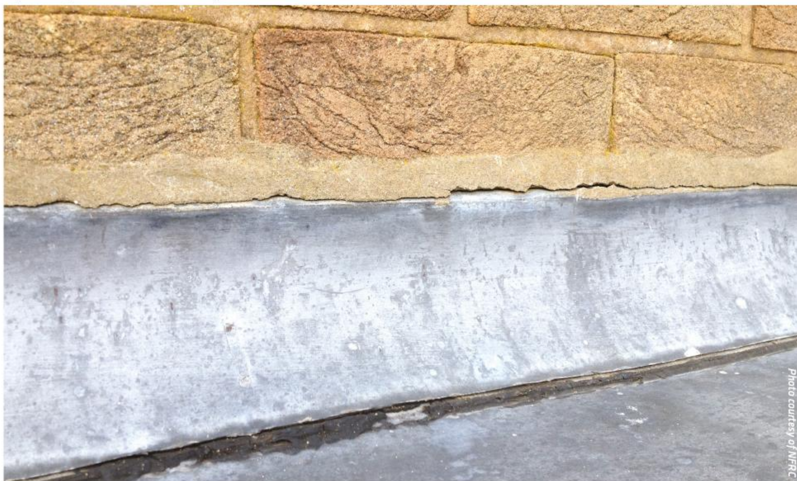
Below: Mortar pointing cracking to lead cap flashing
