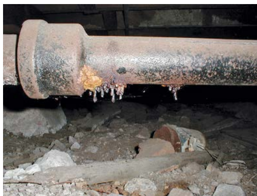
If a cast-iron waste pipe is this rusty, it needs replacing.
