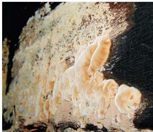
Poor ventilation and a damp dirt floor helped this gaudy fungus blossom on a crawlspace joist. The same conditions encouraged mold to flourish behind the baseboards on the floor above.
