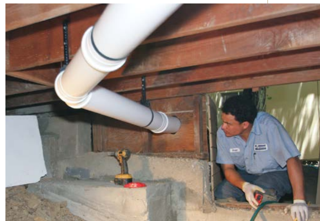
The 5-in. concentric pipe shown here pitches slightly downward toward an exterior wall so combustion condensation will drain away from the heater.
