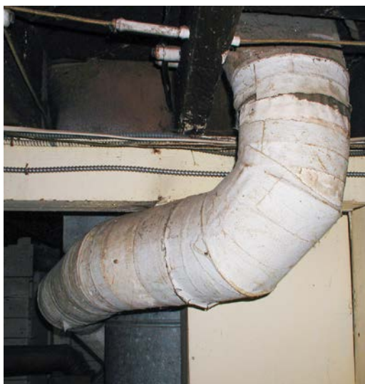
Asbestos is a common wrap on older heating system ducts.
