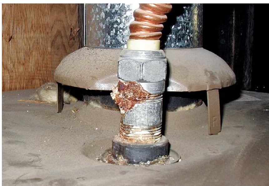
Corroded galvanized-steel pipe atop a water heater tells you it’s time to replace both the heater and the supply pipes.
