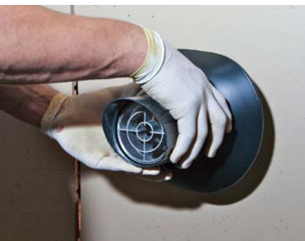
On the outside, the end of the vent pipe is covered by a rubber flange.
