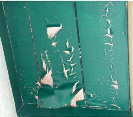
Old wood frequently contain lead paint, which can become an airborne hazard if the paint is sanded or becomes loose.
