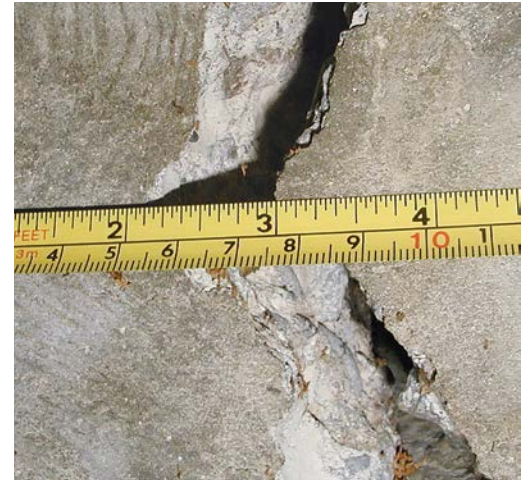
Any crack that runs through a foundation is serious.
