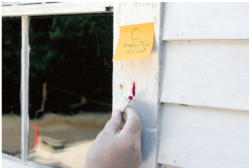
Houses built before 1978 should be tested for lead paint. Cut out a small chunk of surface paint to expose older paint layers, and rub the exposed area with a test swab. This bright-red LeadCheck reading indicates a high concentration of lead.
