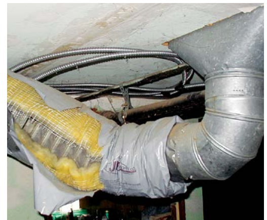
Poorly supported, shedding insulation, and leaking air, this duct should be replaced. Low spots in sagging ducts can become reservoirs for condensation and mold.
