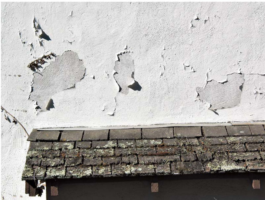
Sheet peeling is caused by excessive moisture migrating through a wall—in this case, an unvented bathroom wall.
