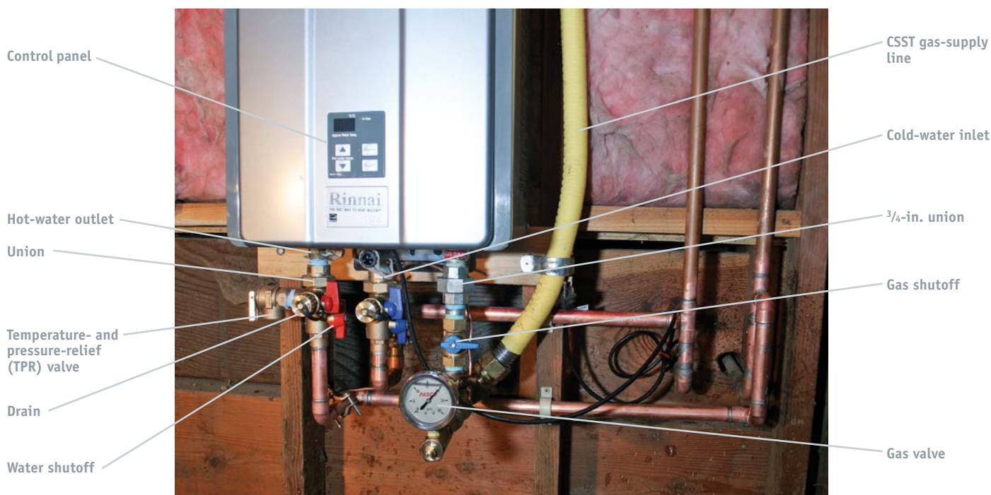
A close-up of connections.
