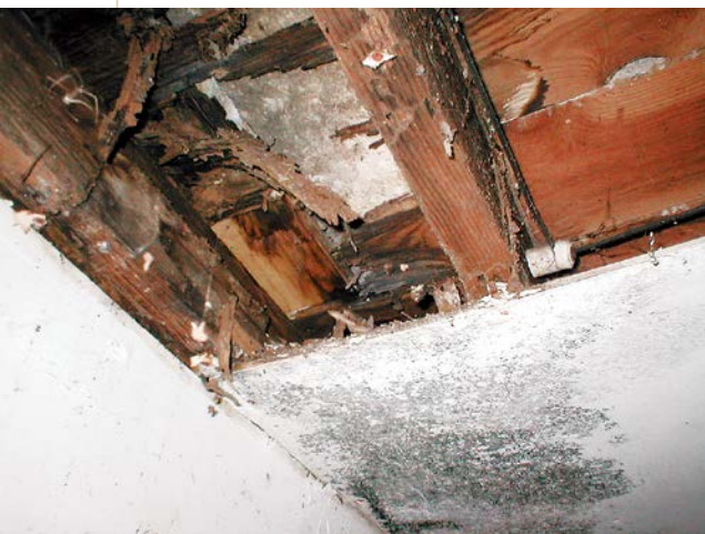
Here, rafter rot, mildewed ceilings, and delaminating roof sheathing were largely caused by inadequate ventilation.
