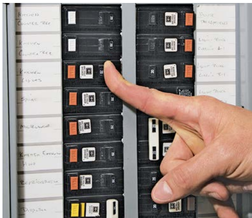
In a breaker box, simply flip the relevant breaker to the off position.
