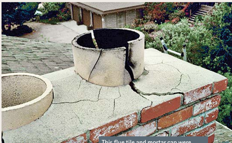
This flue tile and mortar cap were cracked by a chimney fire in a flue that was overdue for cleaning.
