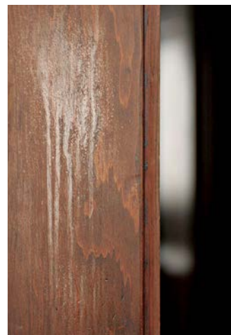
Wax buildup is characterized by uneven, shiny sections where sprayed-on wax has run.
