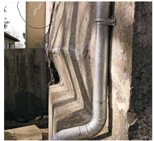
The base of this wall was kicked out by a rotating foundation.
