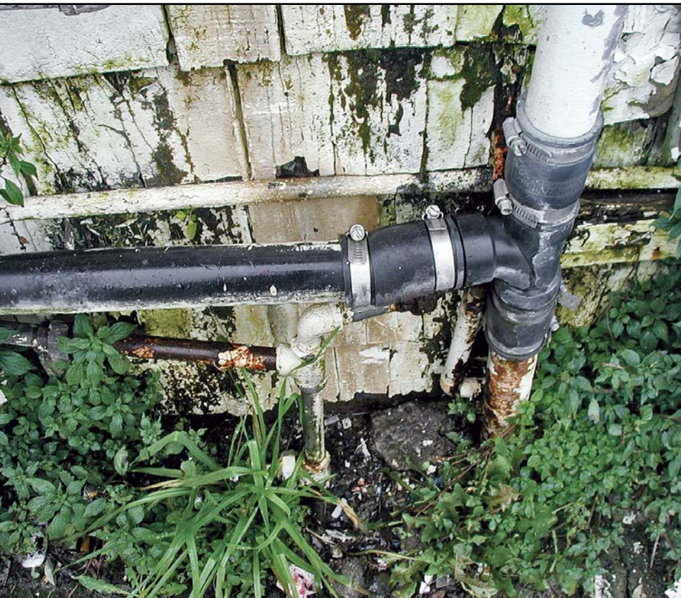
Leaking pipes and vegetation too close to the house were factors in causing this siding to rot.
