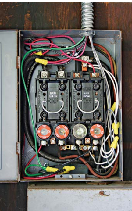
An older fuse box.
