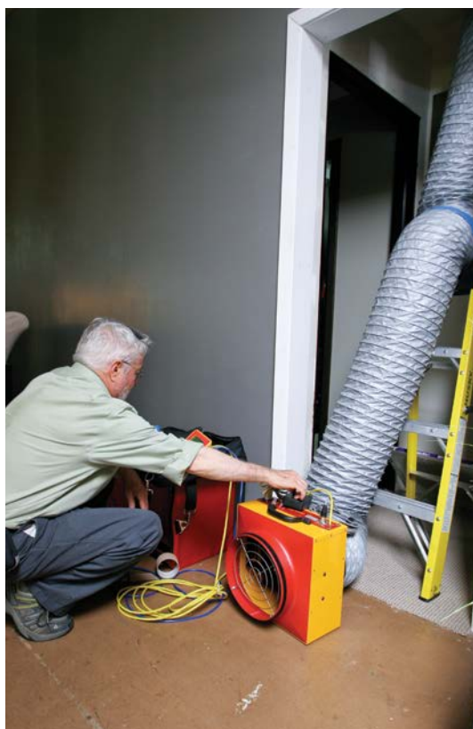
Leaky ducts in a forced hot-air system can squander energy. After sealing heat registers and air intakes, an energy auditor uses a fan to pressurize the ductwork, sometimes blowing theatrical smoke as well, so technicians can see just where ducts are leaking.
