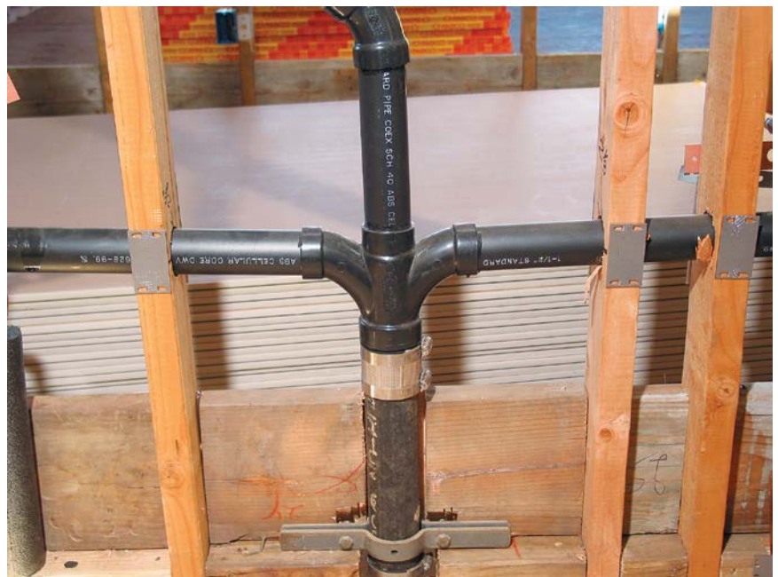
Here, two horizontal ABS lavatory drains meet at a figure-5 fitting, also called a double combo. An ABS vent rises out of the fitting's top hub, while the drain hub connects to a cast-iron stack via a no-hub coupling. A riser clamp supports the bottom of the cast-iron pipe, and steel nail plates protect the ABS.
