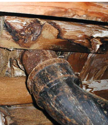
The water damage and rot beneath this toilet could have been avoided by replacing a $2 wax gasket.
