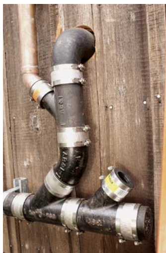
No-hub couplings. At the upper left, a transition coupling joins DWV pipes with different exterior diameters, a 2-in. copper vent pipe, and a 2-in. cast-iron takeoff on a 2 by 3 wye fitting. The other couplings join 3-in. no-hub cast-iron fittings.
