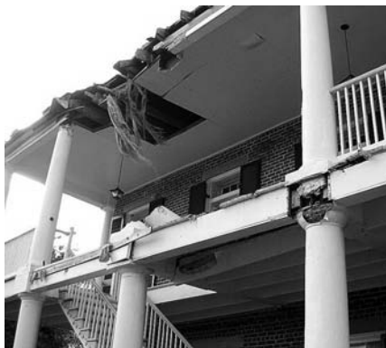
Damage from Hurricane Katrina to an historic building.
