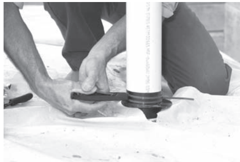
Termite barriers in the basement help keep the pests at bay.
