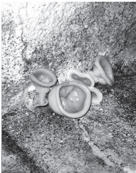
Moisture creates mushrooms on a basement wall.
