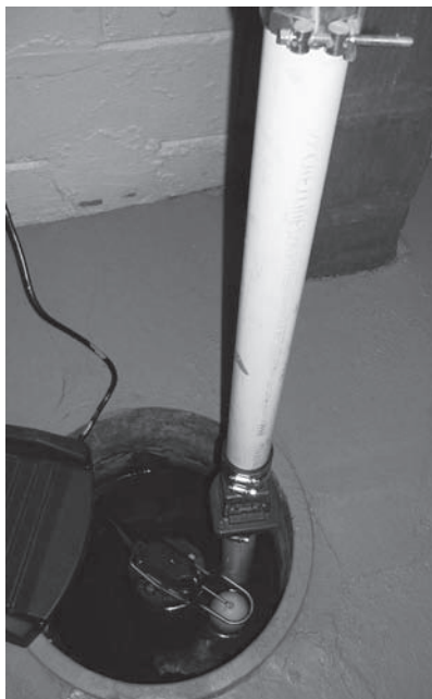
A sump pump in a pit in a basement. The plastic splash block carries water from a drain hole in a dehumidifier collection well so that the well never has to be emptied.
