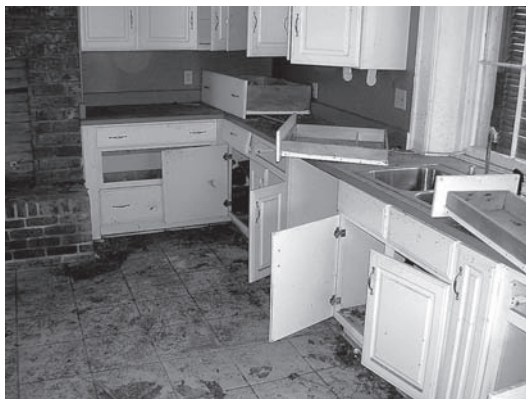
Damage from flooding devastated this kitchen.
