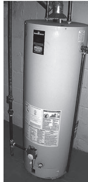
A 50-gallon capacity conventional hot water gas heater in a basement. Most of the energy consumed by these heaters is to keep standing water warm.
