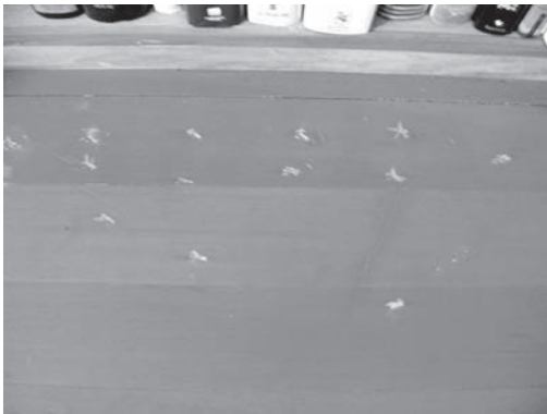
Carpeting was removed from this yellow pine flooring; the underlayment was stapled to the floor, and removing the staples damaged it.
