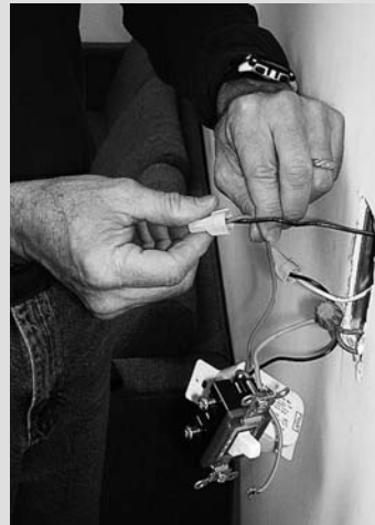
A regular light switch is converted to a motion sensitive one.
