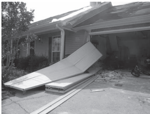
Hurricane-force winds take out a garage door; one-car garages have smaller openings and stand up better.
