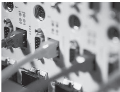
The Ethernet connection to the router.
