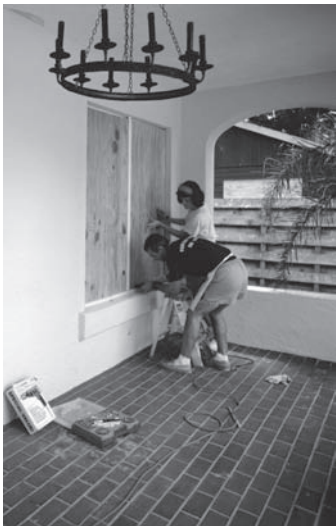
Plywood, if properly installed, protects windows from high winds and projectiles.
