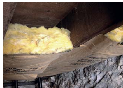
Although stapling a faced batt to the floor joists is easy, this is the wrong way to install fiberglass insulation in floors. Use unfaced batts held with push rods, or insulate the basement walls instead.
