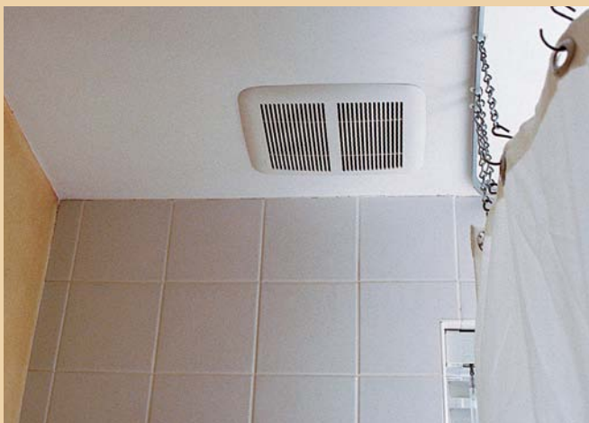
It is important that bathroom fans work properly and exhaust air to the outside, not just into the attic.
