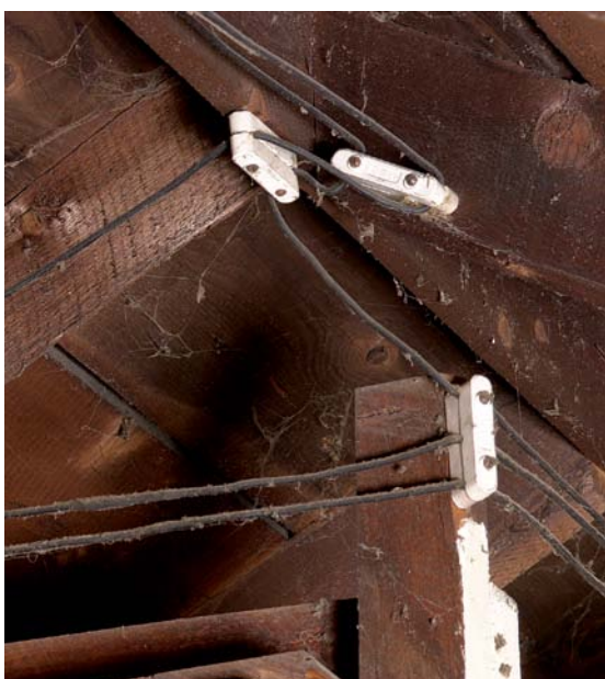
If you have an older house with knob-and-tube wiring that looks something like this, the wiring must be replaced in the attic or wall areas you intend to insulate. To make sure there's no active knob-and-tube wiring hidden in wall cavities, you may want to hire an electrician to verify that it's inactive.
