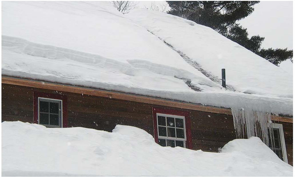
The plumbing wall in this house opens into the cathedral ceiling, dumping warm air into the roof cavity above and melting snow to cause this ice dam.
