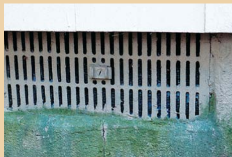
Crawlspace vents do little to reduce moisture in the living space, and they can introduce warm humid air into the crawlspace in the summer.
