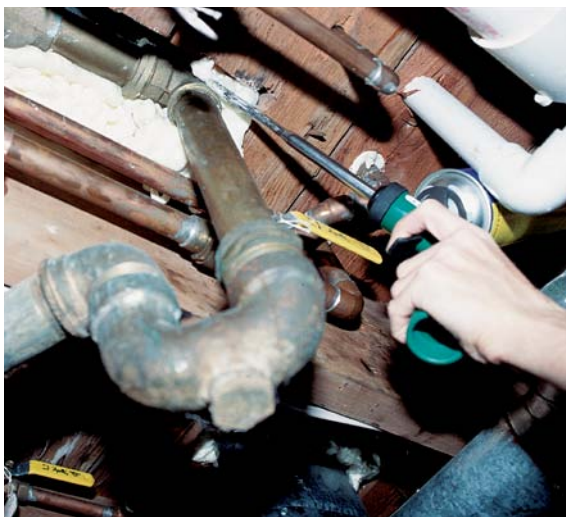
This tub trap is a big air leak from the basement into the house. Note that the duct chase (another big air leak) in the lower right corner should also be sealed.
