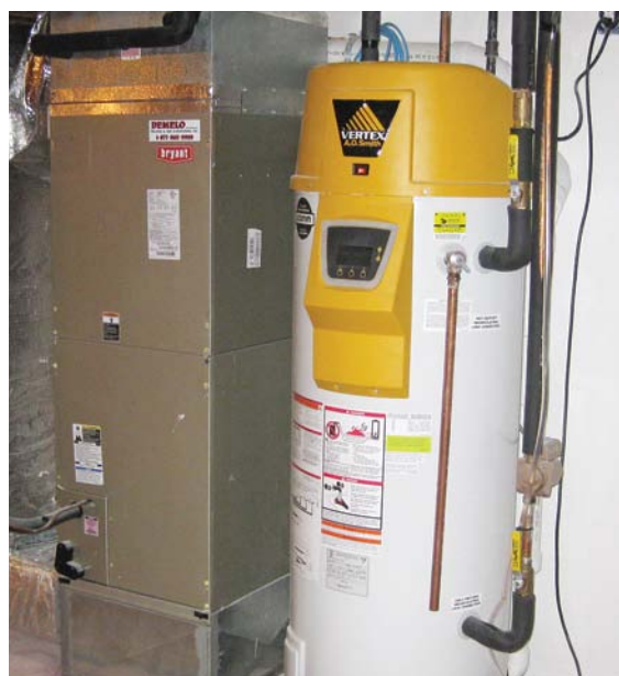
This single, high-efficiency water heater, a Vertex™ by Smith®, has plenty of heat capacity to provide all the heat and hot water for this well-insulated remodel. The box at left is a hydro-air handler, which delivers heat from the Vertex or air-conditioning from an outdoor condenser to a small central duct system.
