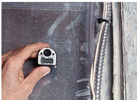
A probe thermometer can be used to check the temperature rise in a furnace. Be careful locating holes so that you don't drill into the air-conditioning coil.
