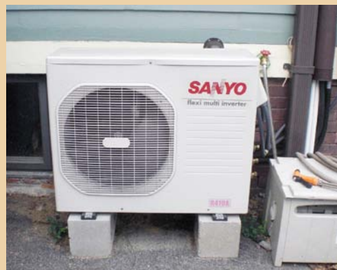
The outdoor half of a ductless mini-split is also small and quiet. I was standing right next to this one and didn't even notice it was running.
