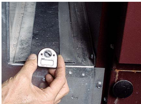
Check the return temperature through a filter slot or a hole drilled in the duct near the air handler.
