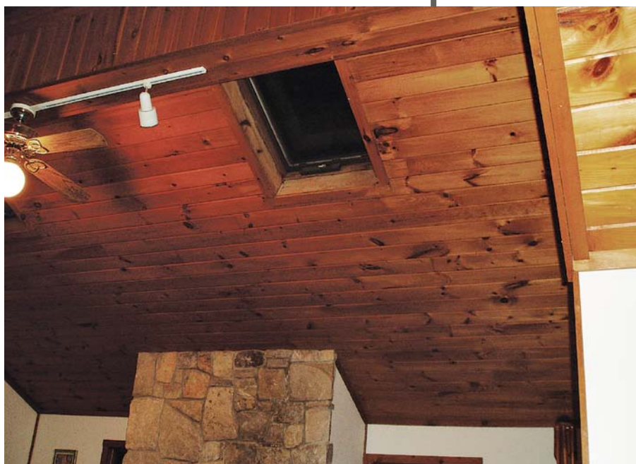
This tongue-and-groove ceiling allows lots of indoor air to reach the cold roof sheathing in winter, where it freezes; when the weather warms up, it rains indoors.
