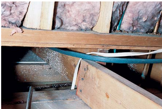
The floor framing behind this kneewall is open right into the attic. Unless these gaps are blocked, outdoor air will circulate between the first and second floors.
