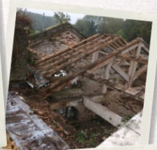
The rear of the house was close to collapse.
