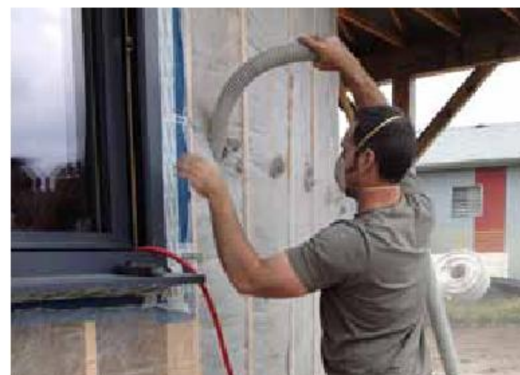
Cellulose insulation actually sequesters carbon, and offers competitive R-values and costs. It can be dense-packed into walls and loose blown into attics.
