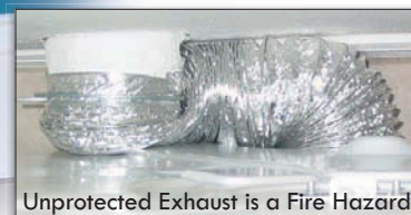
Unprotected Exhaust is a Fire Hazard
