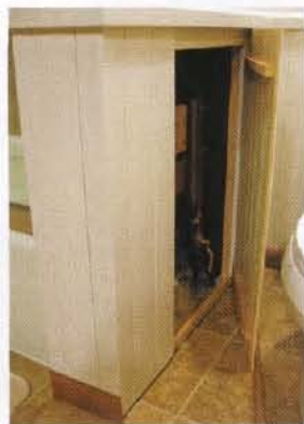
Now you see it, now you don't. The plumbing access makes repairs painless. When closed, the door blends right in.
