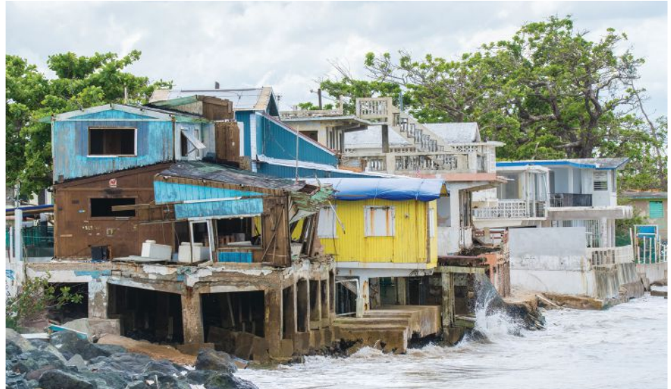
Damage from Hurricane Maria in 2017.
