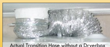
Actual Transition Hose without a Dryerbox
