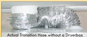
Actual Transition Hose without a Dryerbox
