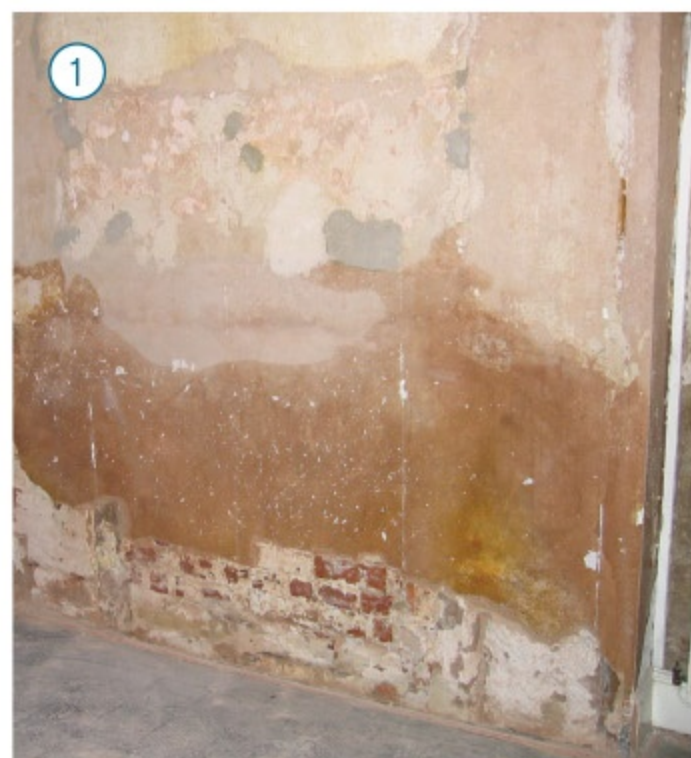
1 Very damp modern plaster covering the bricked-up rear fireplace 2 The fireplace opened up and the surround replastered in lime
