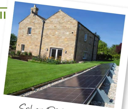
Solar PV panels
