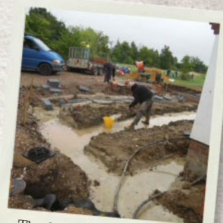
The foundations had to be bailed out after heavy rain.
