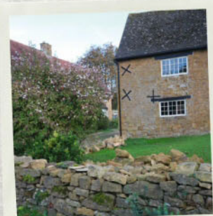
The drystone boundary wall was in need of repair.
