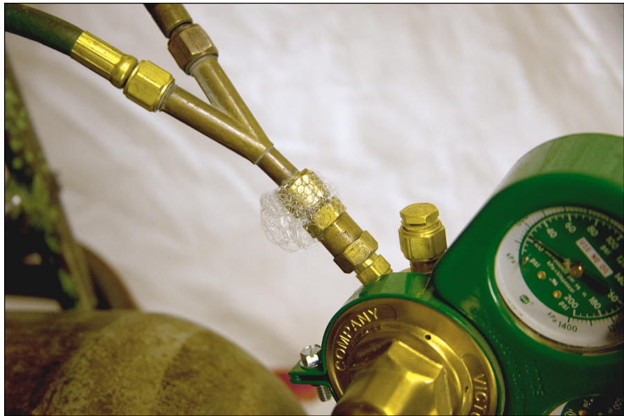
FIGURE 3-4: An example of a leaking oxygen hose.
