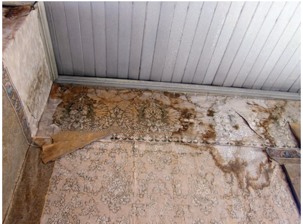
▲ Figure 5.2 Damp in a building
