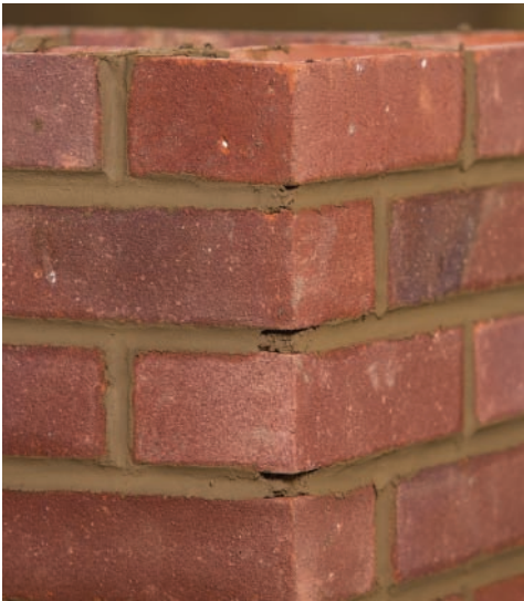
▲ Figure 4.37 Poorly jointed work at the corners of a brick quoin
