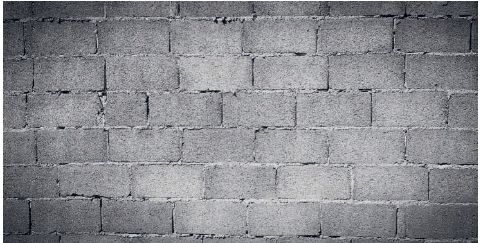
▲ Figure 3.22 A poorly bonded block wall
