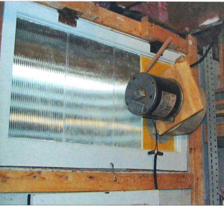
1-7. This exhaust fan is in a window well; a lever raises the well cover when the fan is turned on. I have found that this type is the most efficient in the moving of air. The other advantages are that they are relatively quiet and restrict pests from entering through the opening.
