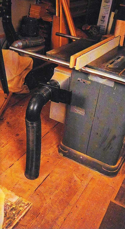
John MacKenzie has underfloor dust collection ductwork.
