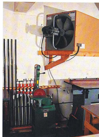
Air circulation and ventilation are critical in Dean Bershaw's basement woodshop. The only direct access to the outside is an opening to a 5" space between building walls. He built a diagonally mounted fan housing so that air could be exhausted into the narrow space between buildings.
