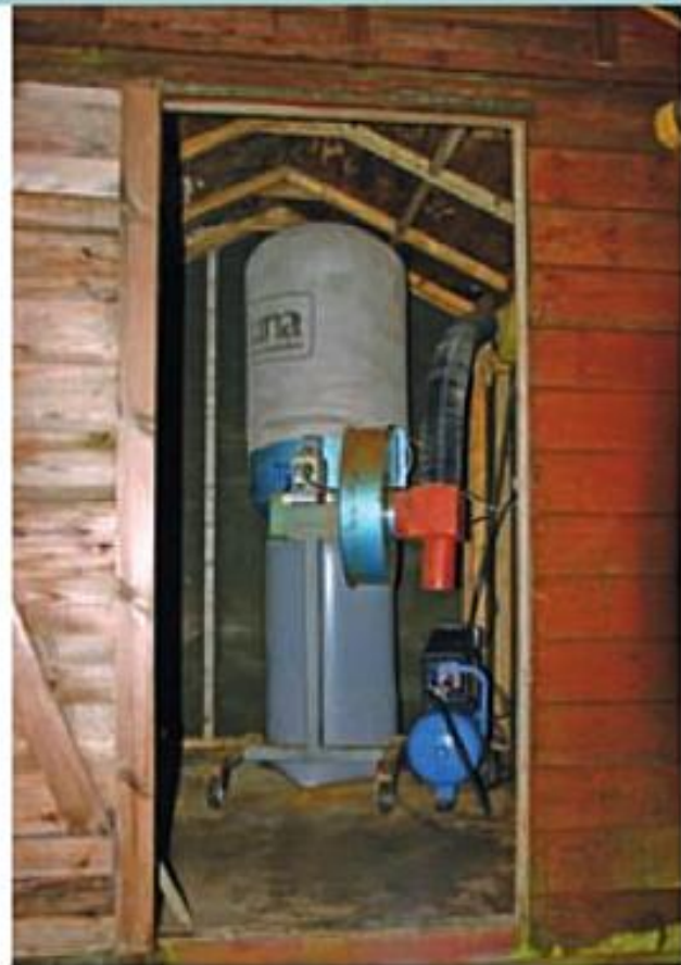
Above Double-bag chip extractor and compressor in separate shed.
