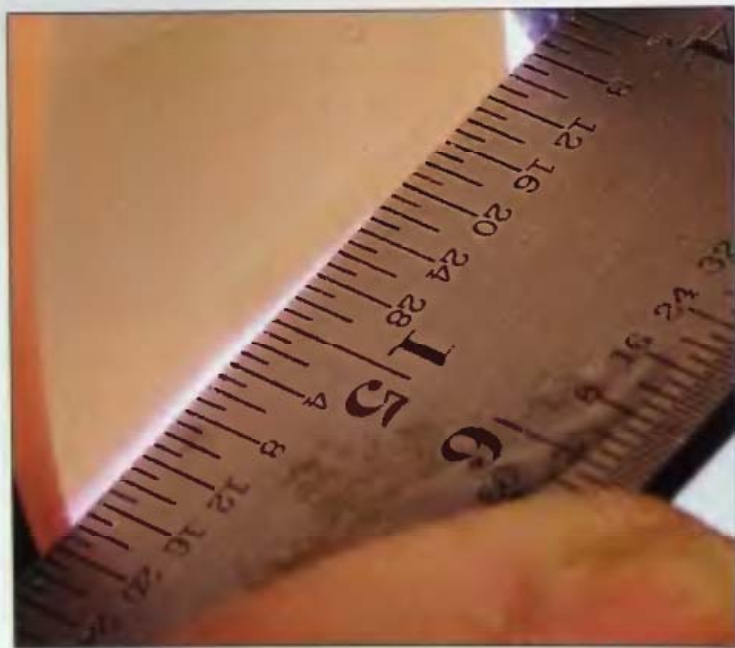
7-26 The flatness of this surface needs improvement.
