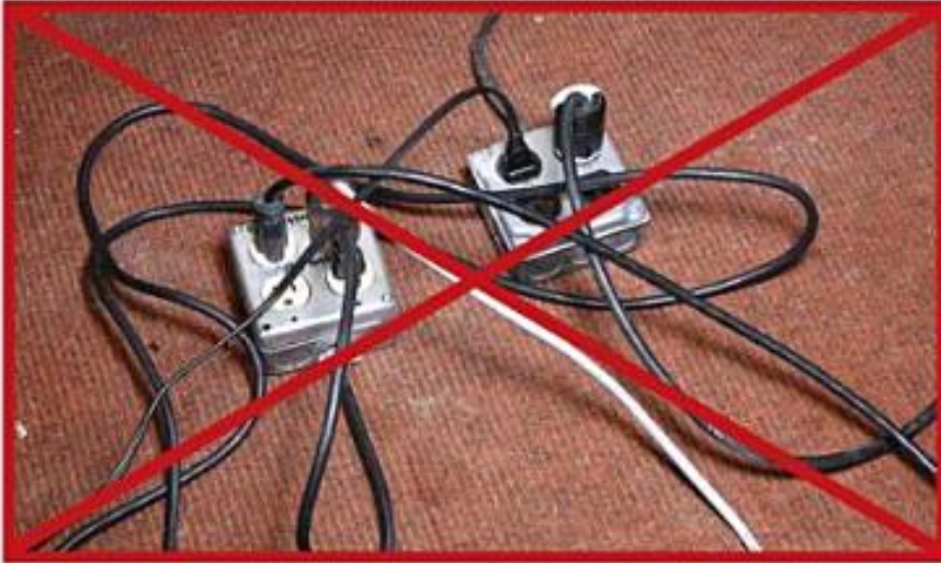
Photo 1.9. Avoid situations in which power cords can be a tripping hazard or can cause an overloaded circuit.
