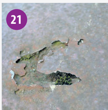
Now to the rear wings, this rot hole is in the top face, it must have rotted from beneath where it is fitted to the support.
