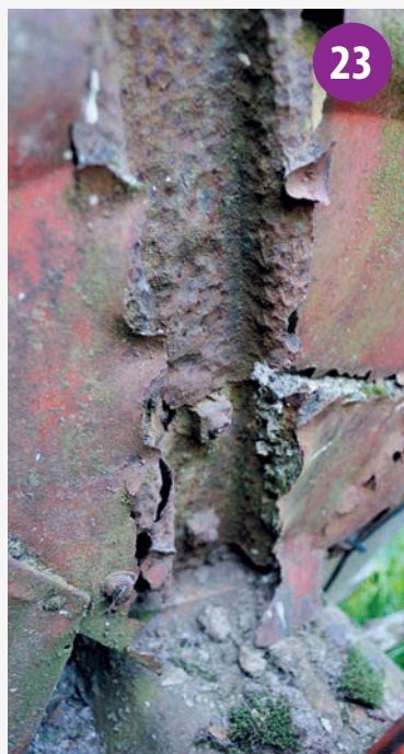
The front support has now cracked off near its base, hence the wing is swinging about.
