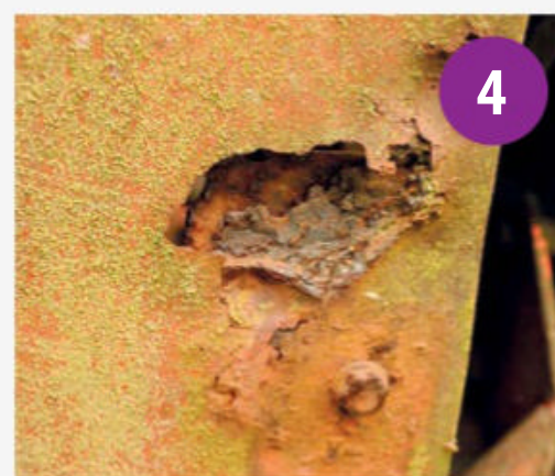
The other side is not much better with rot in the attachment bracket.
