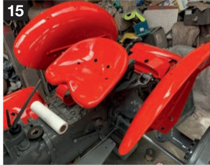
15 I love this part when I can fit the shiny red items on the grey skid unit. These tractors were never this shiny new!
