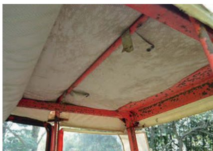
The roof was the same as the door in that it was padded; the front section was falling off because a pole was rotten due to condensation.
