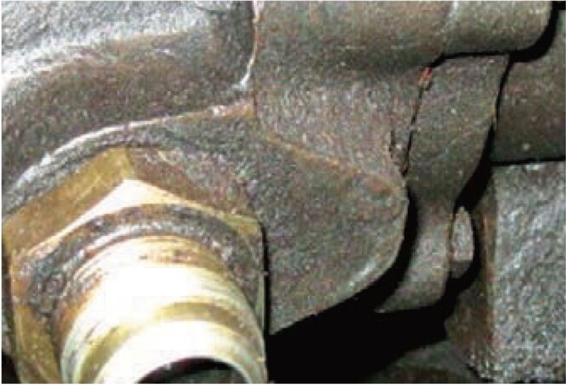
The hydraulic pump was modified years ago to work with threaded nipples instead of push-in pipes. Hydraulic hoses have replaced the steel pipes.
