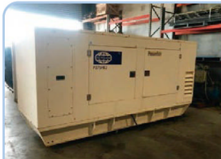
FG WILSON 275KVA DIESEL GENERATOR USED 1796 HOURS
