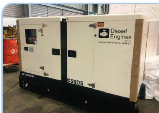
NEW CUMMINS 60KVA GENERATOR 3 PHASE SILENCED
