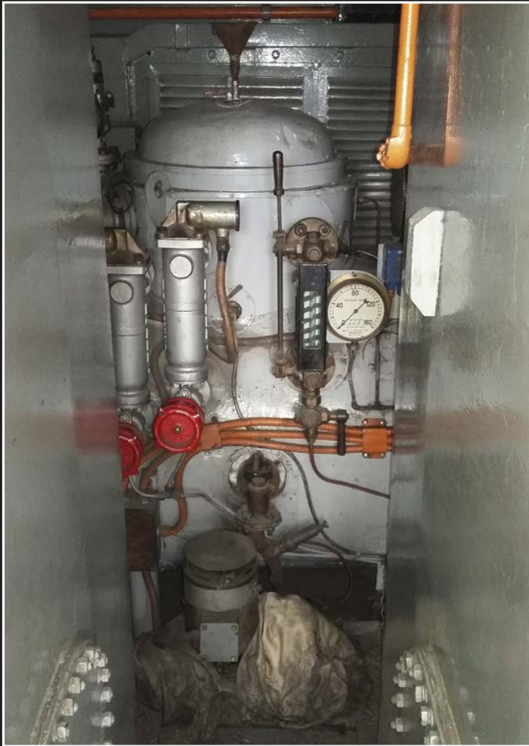
Things are always cramped in the locomotives as shown in this view of a Spanner boiler on preserved 46045. BOB DUNN
