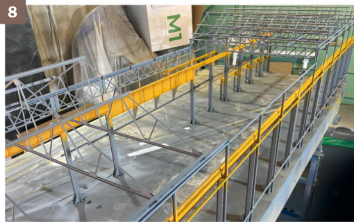
8 ▲ Having established the optimal order for applying the main colours, the first parts were painted, starting with orange on the crane beams, including the beams in the wheel shop.
