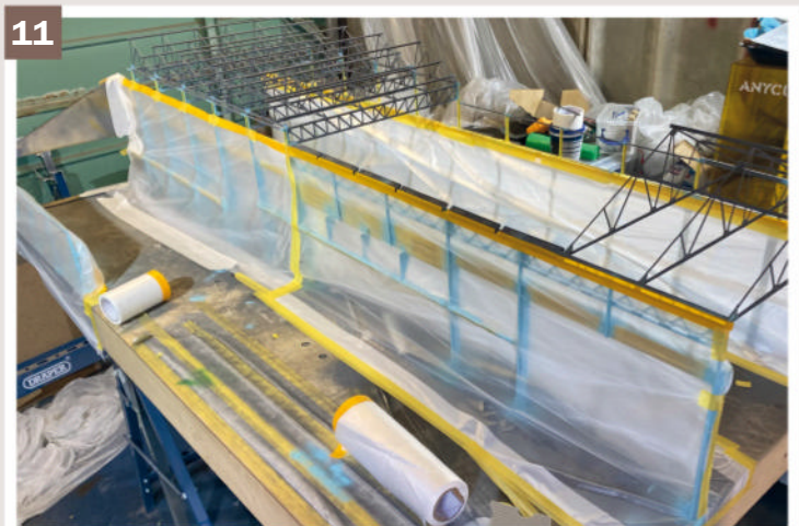
11 ▲ With the side structures of the erecting shop painted, these were masked off to next tackle the roof trusses and north light frames. Polythene sheet was used.
