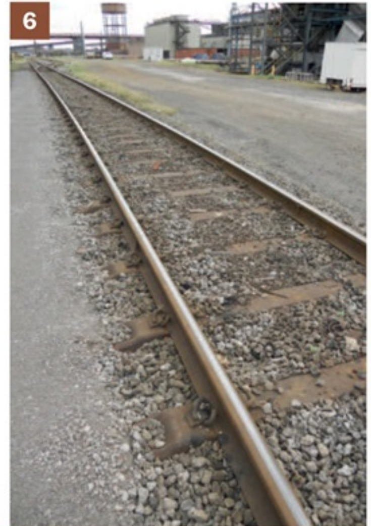
Pandrol channels were substantially stronger than the Wisclip version and better at retaining the rail in place.
