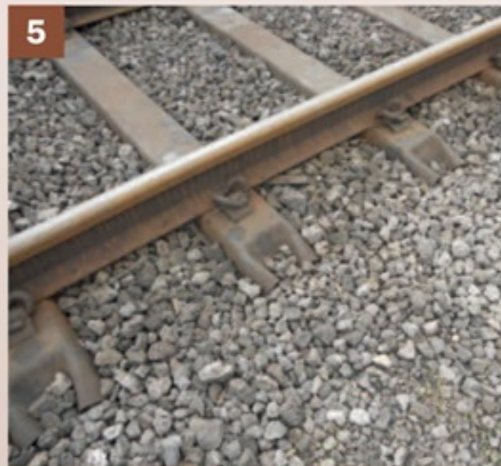
Pandrol channels were introduced following instances of cracking beneath the foot of the rail.
