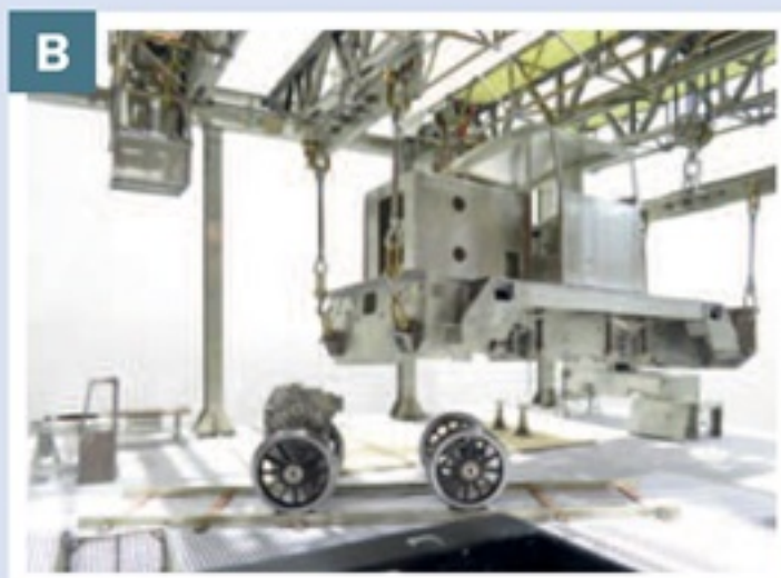
▲ The cranes traverse across the shop for positioning over the wheelsets.
